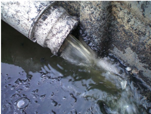
Picture 4: effluent during dewatering mode
