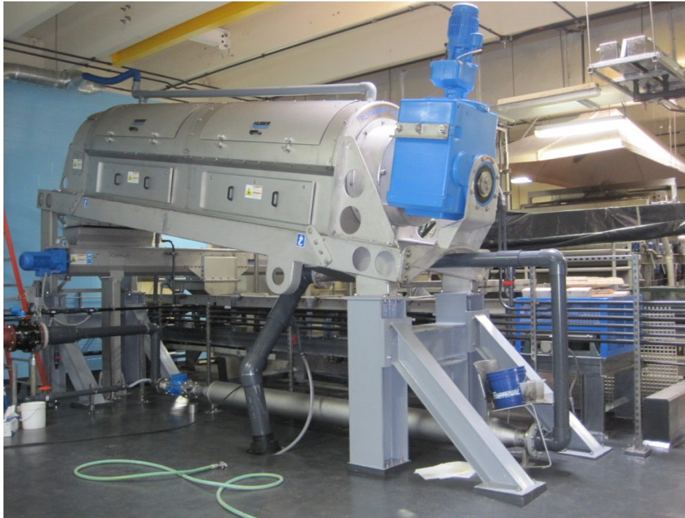
Figure 7: Huber Screw Press at the Lakehaven Utility District's Lakota Wastewater Treatment Plant
