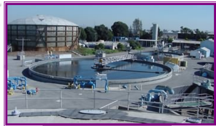
Wastewater pretreatment plant.
