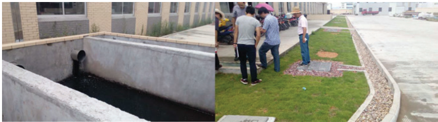
Figure 8.8 Rainwater harvesting system: pre-treatment and storage tank.
