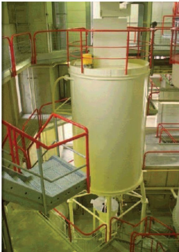
Figure 10 - Seeding sand storage silo with sand washer underneath
