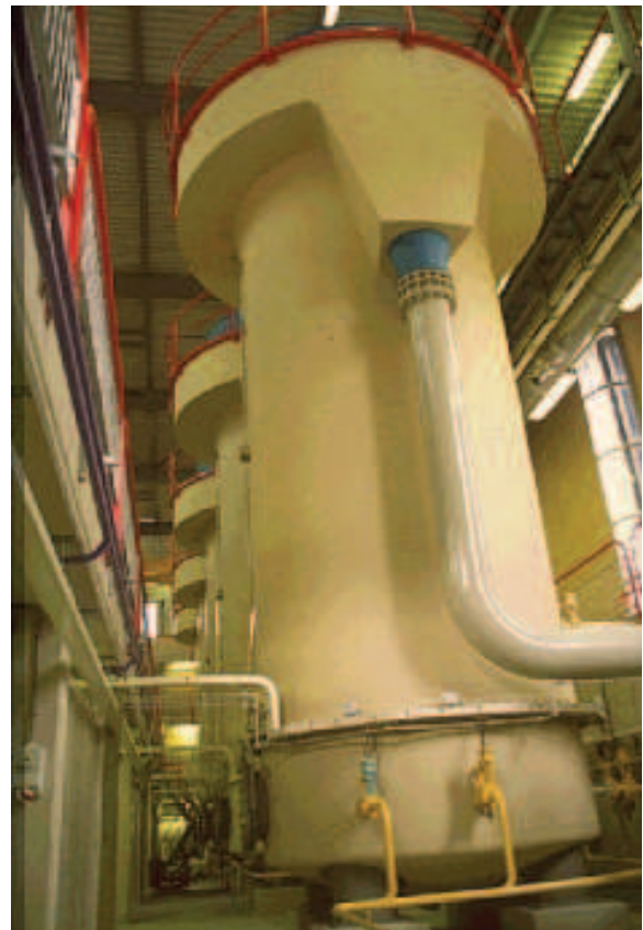
Figure 1 - Pellet reactor used for softening of drinking water
