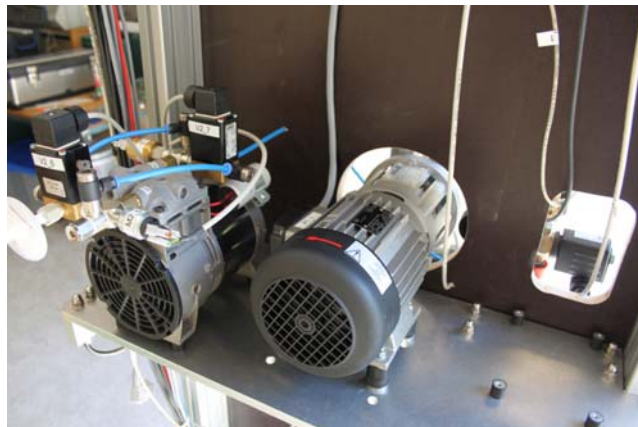
Figure 4.8 Circulation pump of 1st stage and vacuum pump for draining 1st stage and transferring to 2nd stage.
