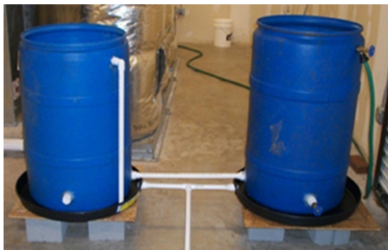
Figure 9.8 Condensate holding tanks and irrigation pump.
