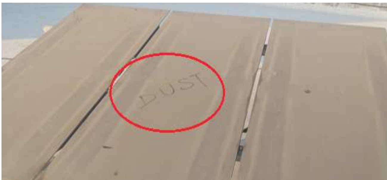
Figure 25: Cleaning required (Significant financial impact)
