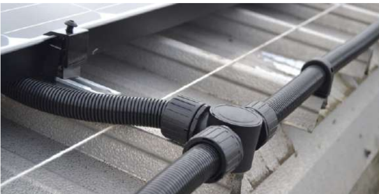
Figure 110: Correct - Conduits are in proper condition
