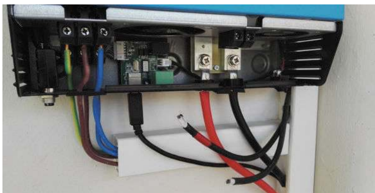
Figure 83: Disconnected wire from inverter base
