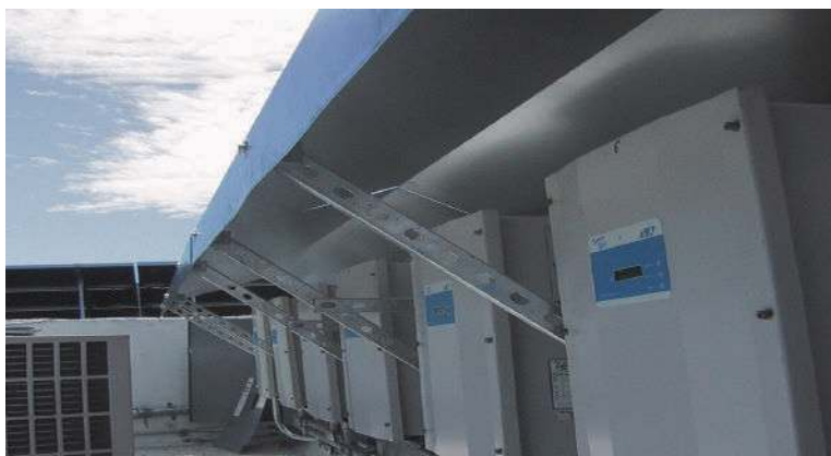
Figure 85: Inverter installed under shade
