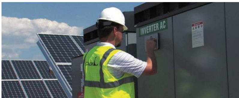
Figure 78: Note readings from inverter display screen
