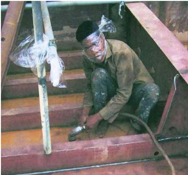
Figure 154: Incorrect practice - Without face shield
