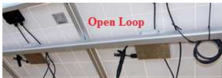
Figure 103: Incorrect cables connection looped loosely
