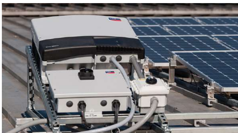
Figure 84: Inverter installed without any shade or roof
