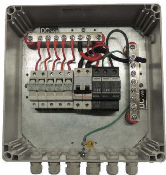
Figure 8: Strings Junction (SJB)
