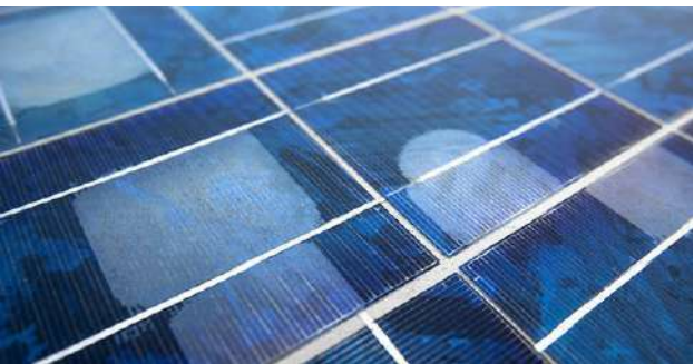
Figure 34: Tiny Hairline Cracks
