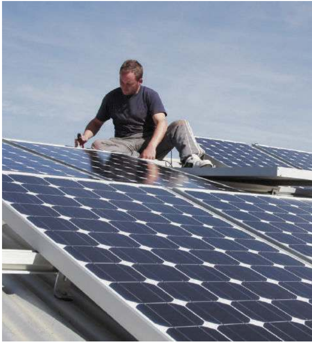
Figure 160: Incorrect practice - Without safety belts
