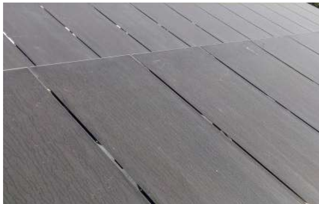
Figure 24: Cleaning Required Shortly (No significant financial impact)
