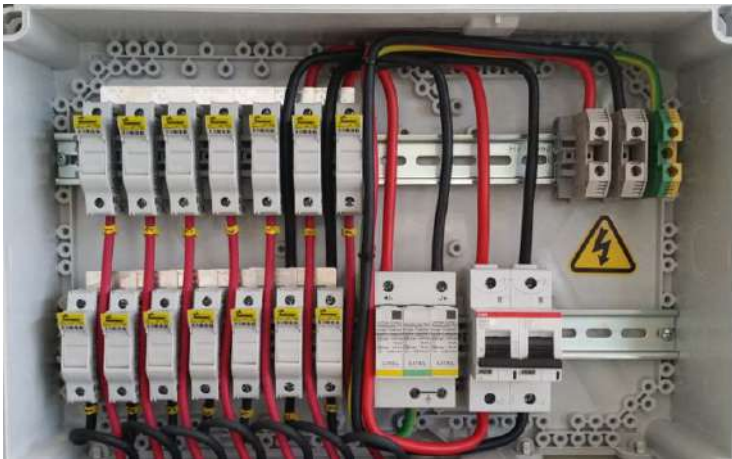
Figure 111: Cables are labelled properly
