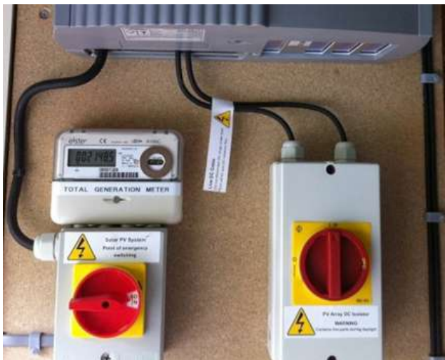
Figure 95: Overcurrent protection devices (OCPDs)
