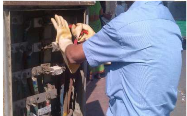
Figure 159: Correct practice - With safety gloves
