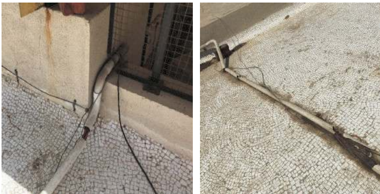
Figure 109: Incorrect - Conduits are damaged
