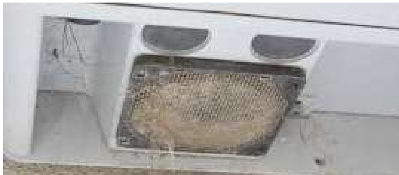
Figure 88: Dust accumulation on Inverter
