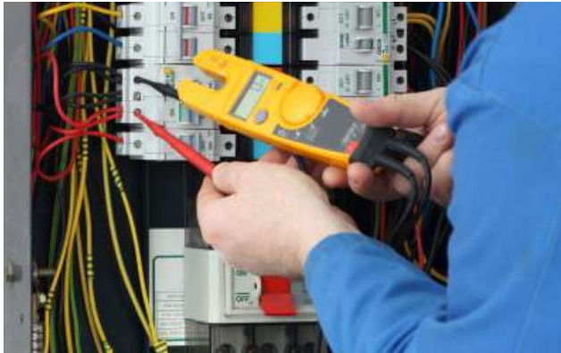
Figure 158: Incorrect practice - Without safety gloves
