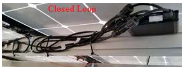
Figure 102: Incorrect cables connection looped tightly
