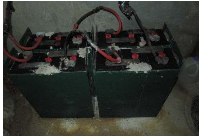
Figure 127: Improper condition of battery
