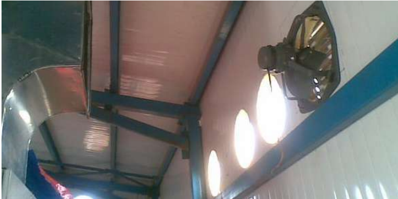
Figure 87: Inverter ventilation room
