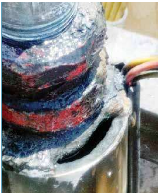
FIGURE 35. Stray electrical currents formed a hole in this submersible pump. Water was forced through the hole in the bottom of the pump, causing the well screen to collapse and the well system to fail. (Source: Mike Prestigiacomio)
