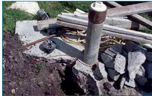
FIGURE 59. The slab around this well is not sufficient to prevent surface contaminants from entering the aquifer. (Source: Plugging Abandoned Water Wells , Bruce Lesikar and Justin Mechell, 2010.)
