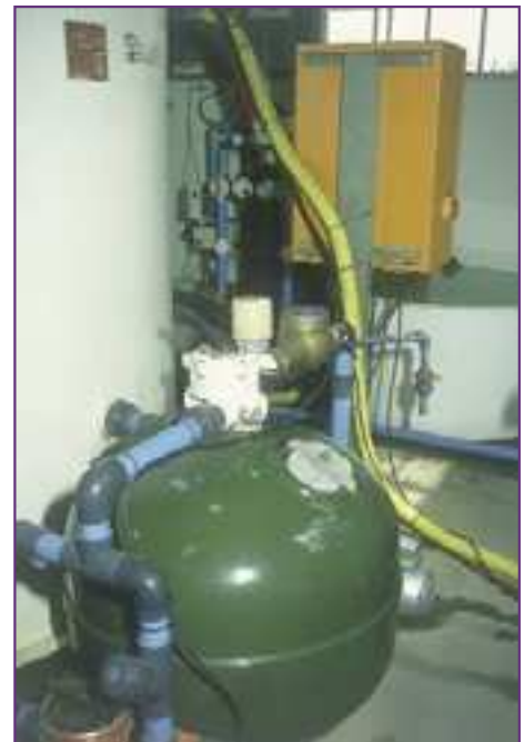
Figure 13: Small-scale pressure sand filter
