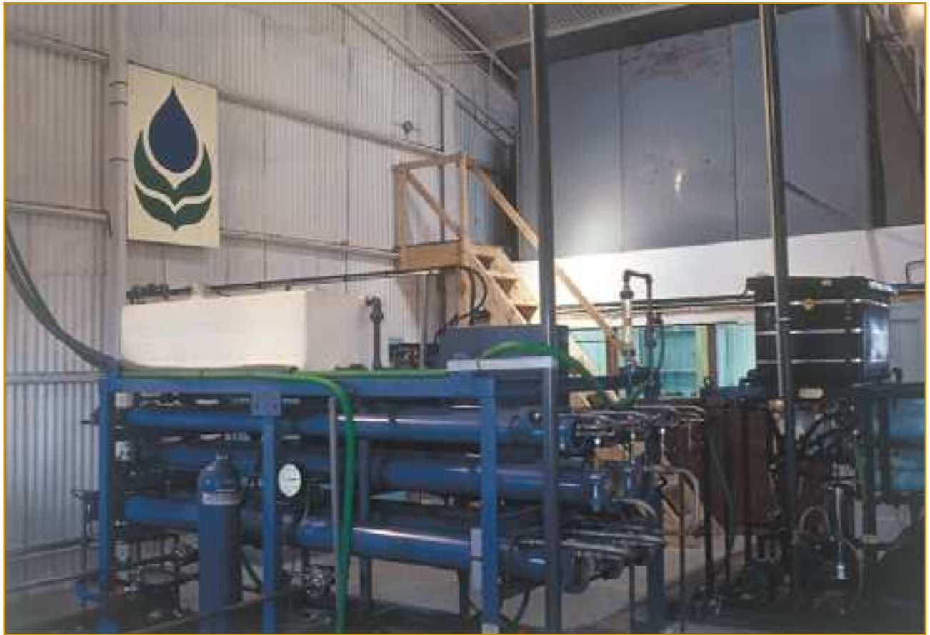
Figure 5: Specialised reverse osmosis desalination plant
