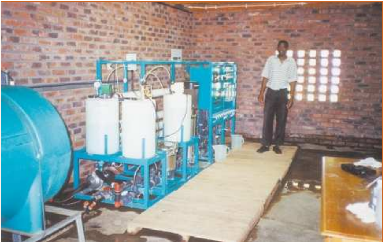
Figure 18: Small-scale RO plant
