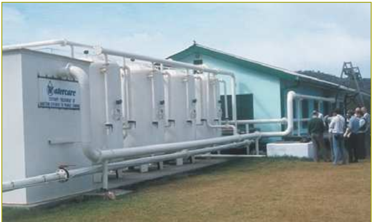
Figure 16: General view of package treatment plant
