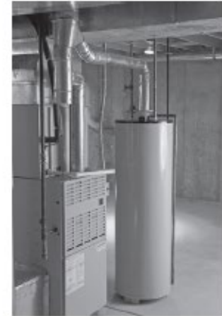
Heating systems (© Comstock RF.)
