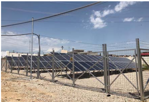
Figure 8.2 Solar-powered water project in Shekhan.
