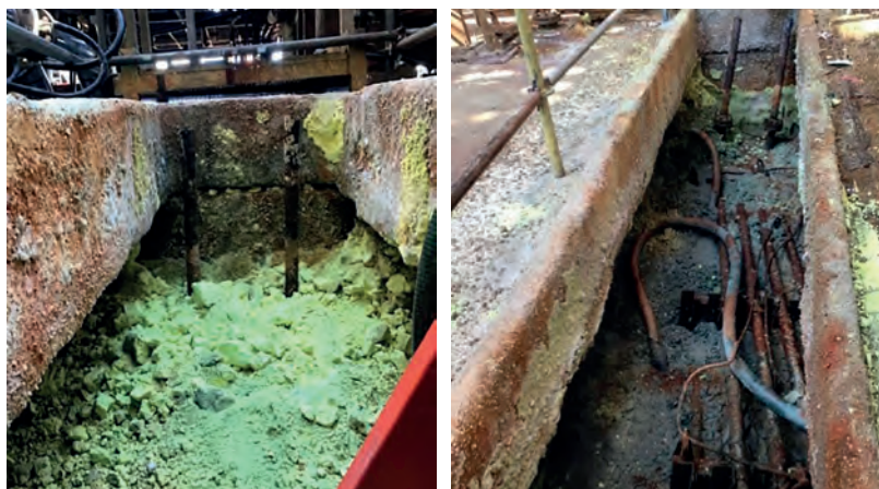
Figure 2. View of a cold sulfur pit filled with solidified sulfur cake at a roof slab portal location (left). The adjacent portal revealed temporary heating coils in-place, with little effect on melting subsurface sulfur cake deposits (right).
