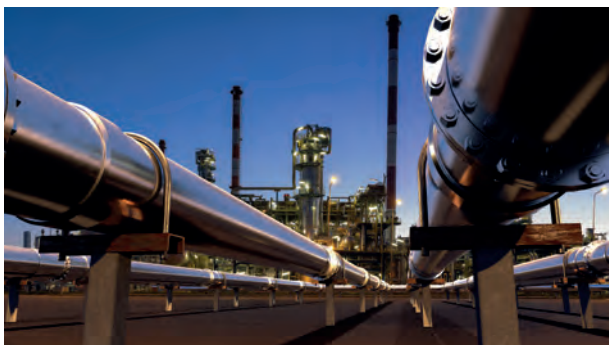
Figure 3. Leveraging AWS for a customised, condition-based maintenance project, a leading Australian natural gas producer reduced the cost of routine inspection and service by 80%.
