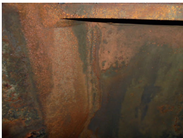
Figure 4. The 2021 inspection of the six columns coated with a low velocity thermal spray shows severe corrosion and risk of failure.
