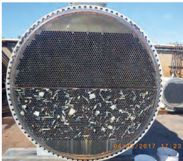
Figure 4. Debris in the inlet of the critical heat exchanger.
