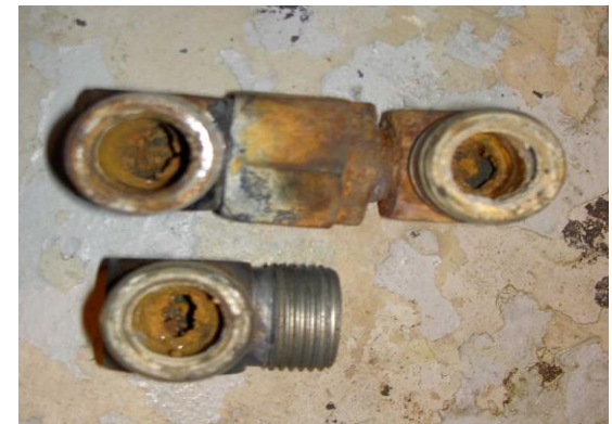
Cooling Tubes Plugged
