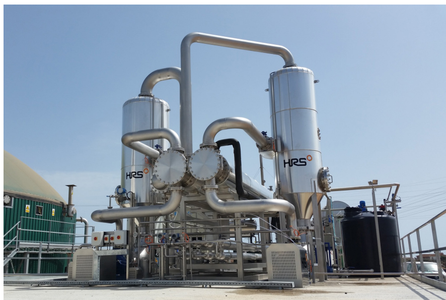
This HRS digestate concentration system in Spain allows the farm-based plant to store its digestate until the most beneficial period for application to land as a biofertilizer.
