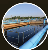
Wastewater Treatment Tanks
