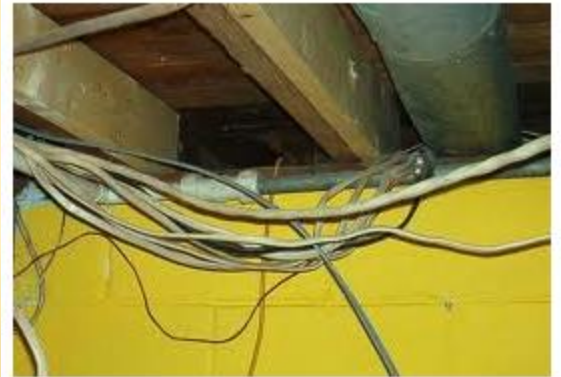
Loose wires and faulty joints
