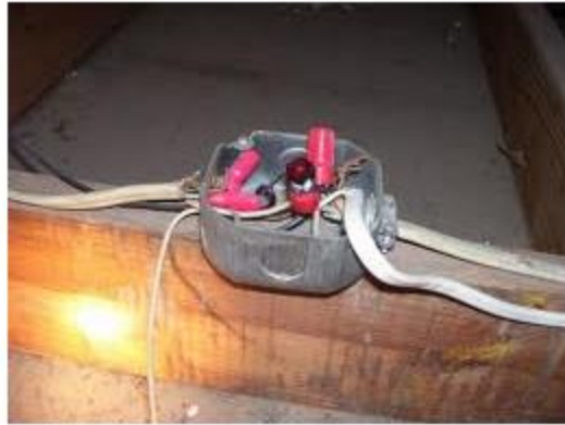
Missing, broken or inadequately secured covers
