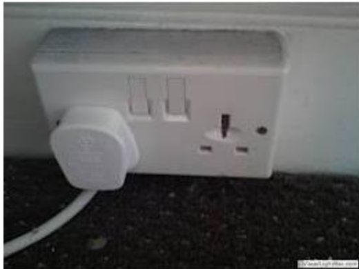
loose or damaged socket outlet
