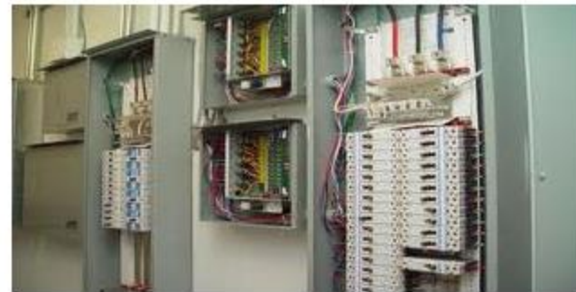
Open or inadequately secured panel doors
