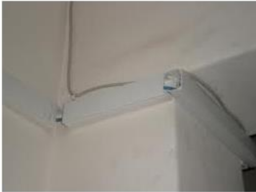
Damaged or loose conduit, trunking and cabling
