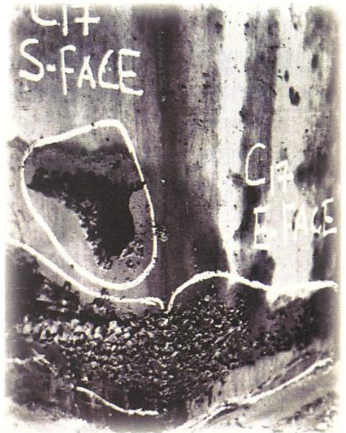
Figure 3 : RCC column displaying porosity due to segregation of concrete whilst placing.
