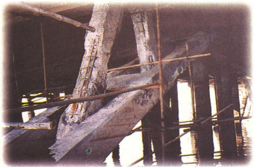
Figure 11 : Trombay jetty showing concrete deterioration in the atmosphere and tidal zone
