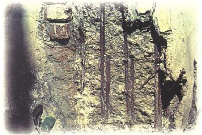
Figure 7 : Spalling of concrete of a building column due to rusting of steel reinforcement.
