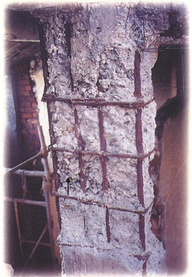
Figure 2 : Column showing porous concrete due to improper mix and incorrect construction practices.
