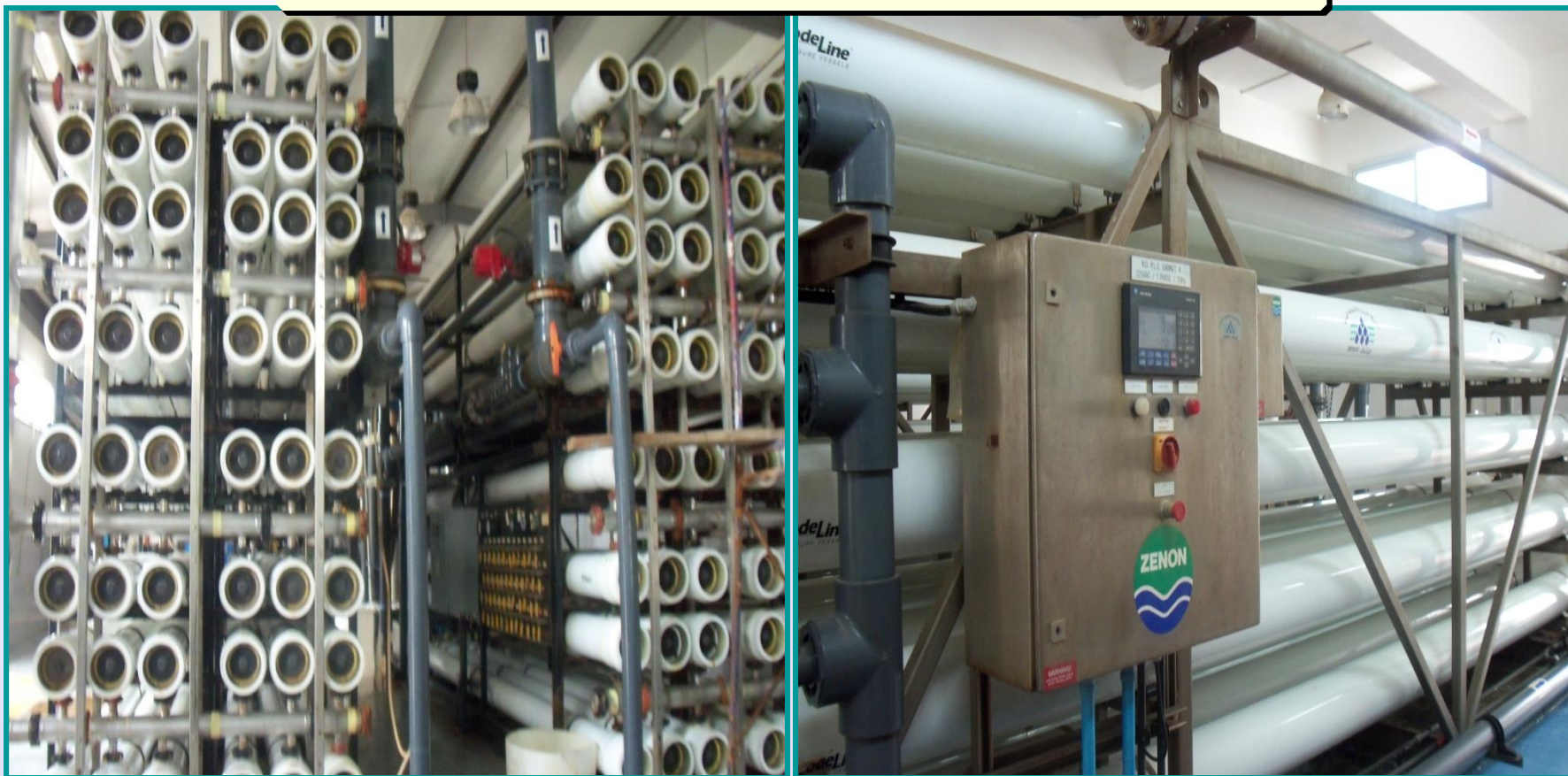
Sharm el shiek Desalination plant ( 10000 m 3 /day )
