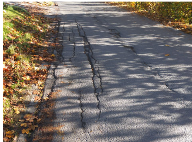
Fig. 8.26 A special type of freeze-thaw erosion is ground frost rising. There are many places, where you can observe this after the damage of the road surface. Fine materials in the road base observe water and these freezes in the winter. The results are easy to observe when the spring comes
