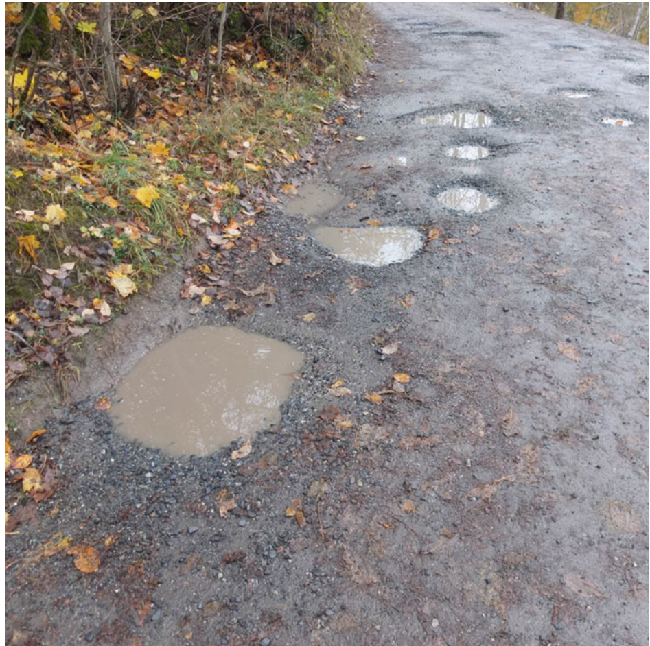
Fig. 8.28 Combinations of water and human activity can be an efficient erosion mechanism
