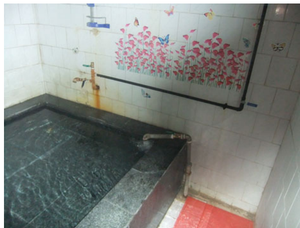
Fig. 10.65 In small bathrooms the visitors in Huaqing Chi can enjoy water with a temperature of 43 °C. The mineral rich water is claimed to have health-bringing effect, and a therapeutic effect on the skin through the mineral and organic compounds. The bathrooms also have massage benches
