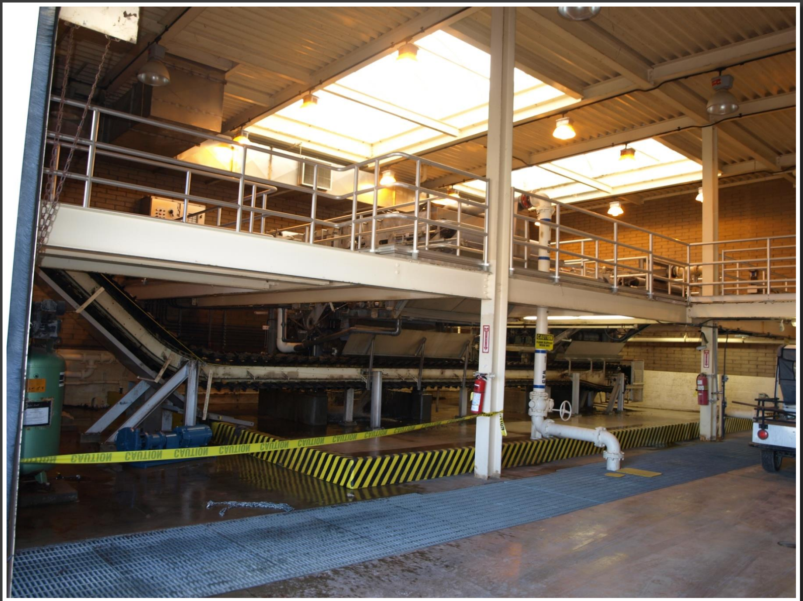
Mechanical drying facility (belt press)
