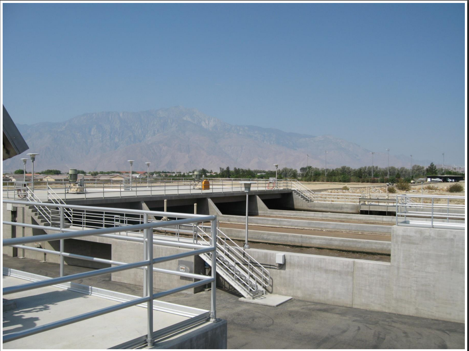
Extended aeration ponds
