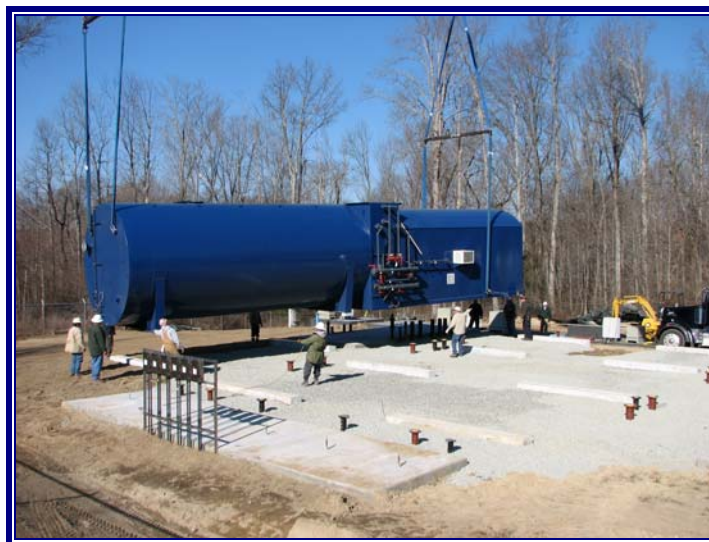
Figure 4. Portability of the MBR Wastewater Treatment System as Demonstrated by Installation Method.
