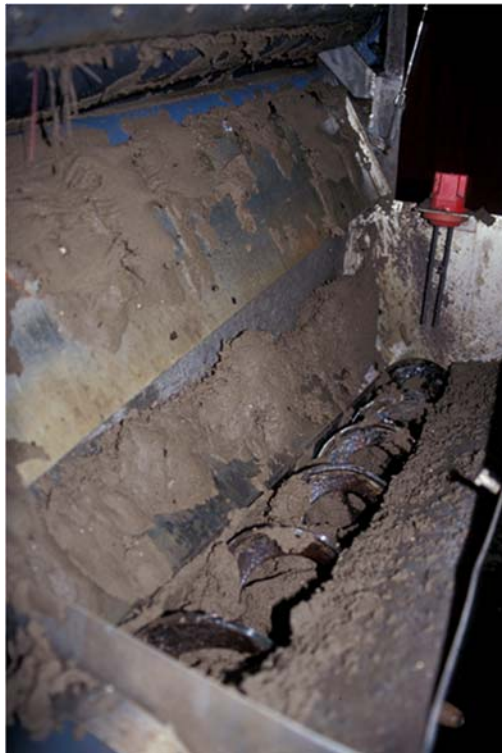
Figure 20. Band filter dewatered sludge outlet.
