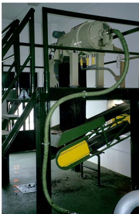
Figure 13. General view of a centrifuge for dewatering.
