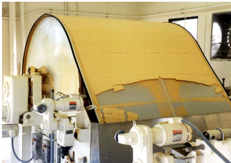
Figure 6. Vaccum filter dewatering.
