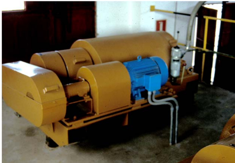
Figure 12. General view of a dewatering centrifuge.
