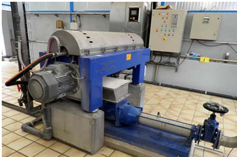
Figure 8. General view of a thickening centrifuge.
