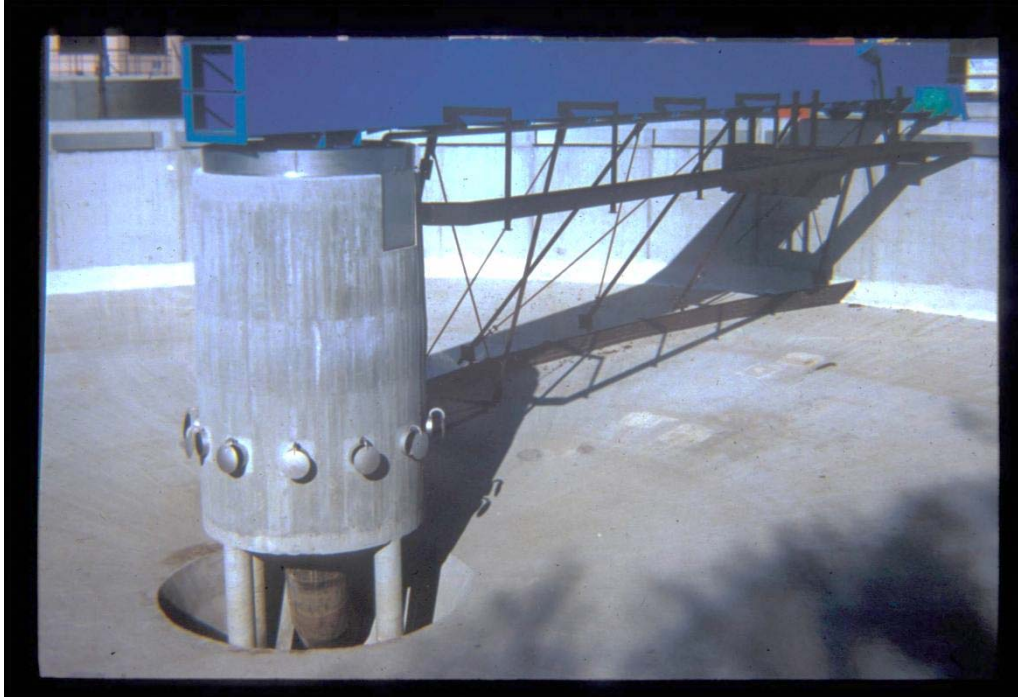
Figure 15 General view of a circular primary clarifier with moving arm and central raw water distribution system
