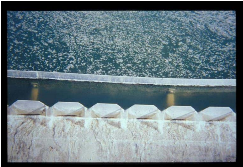
Figure 22 Detail of clarified water over the effluent weir: baffle and v-notch weir.
