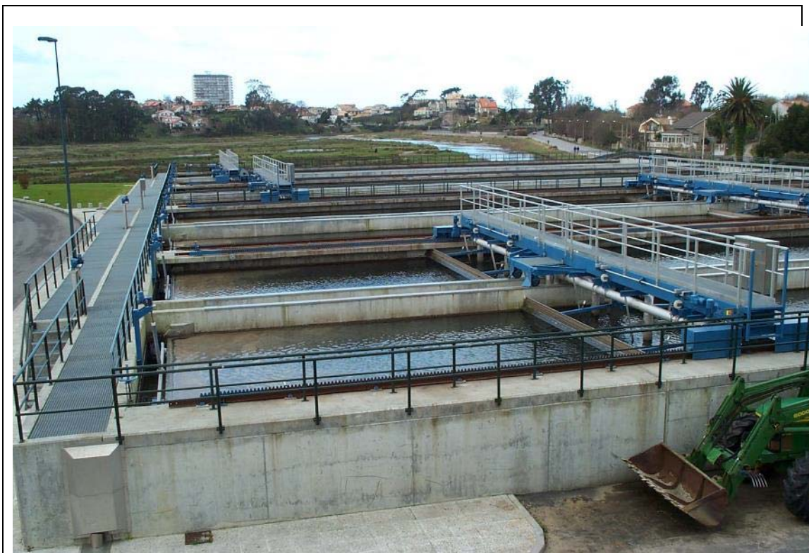
Figure 10 Primary rectangular clarifiers with skimmers fixed to a moving bridge.
