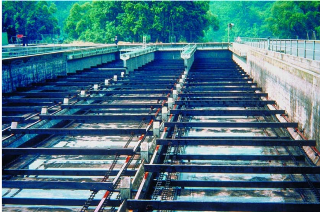
Figure 11 Rectangular clarifier with chain scrapers bottom cleaning system
