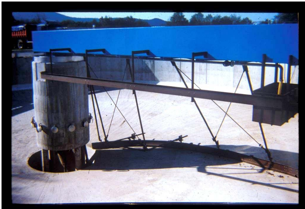
Figure 16 General view of a circular primary clarifier with moving arm and central raw water distribution system
