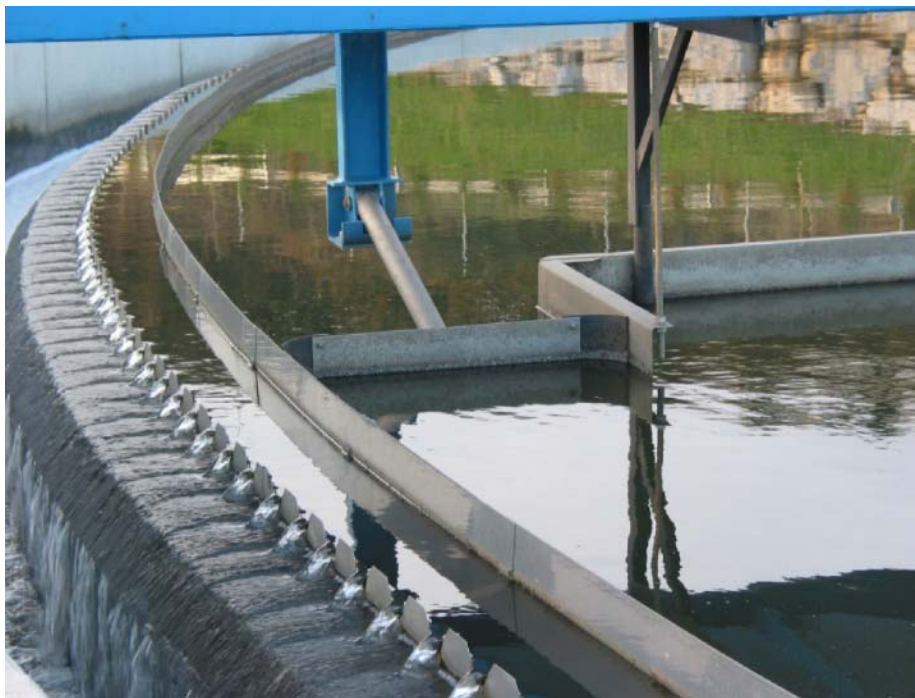
Figure 32 Detail for the clarified water extraction with scrapers system for floating matter removal.
