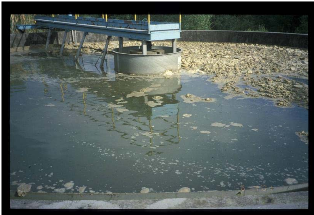
Figure 26 Primary clarifier where sludge floating happened.
