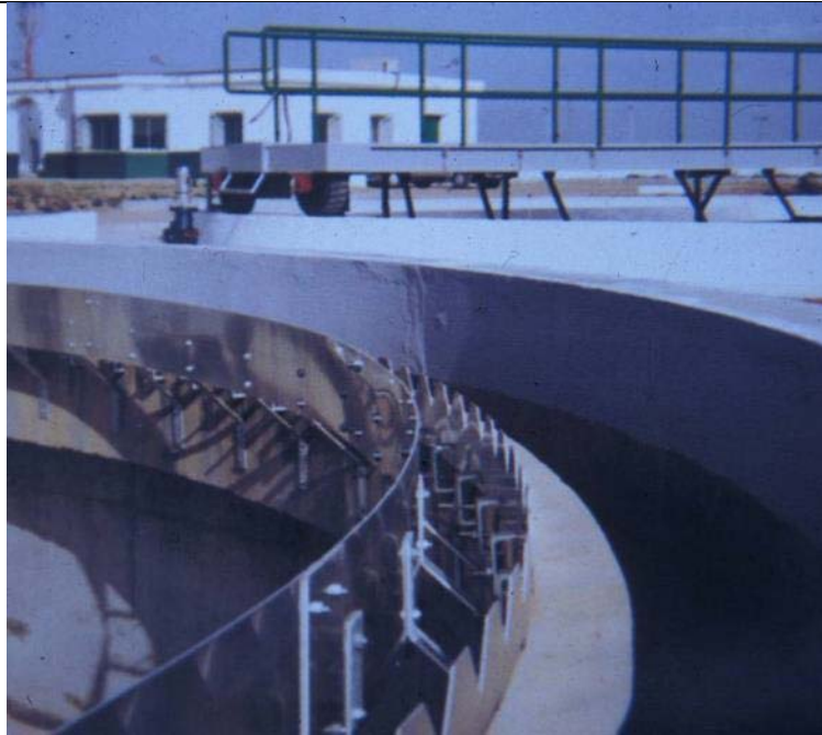
Figure 21 Detail of clarified water over the effluent weir: baffle and v-notch weir.
