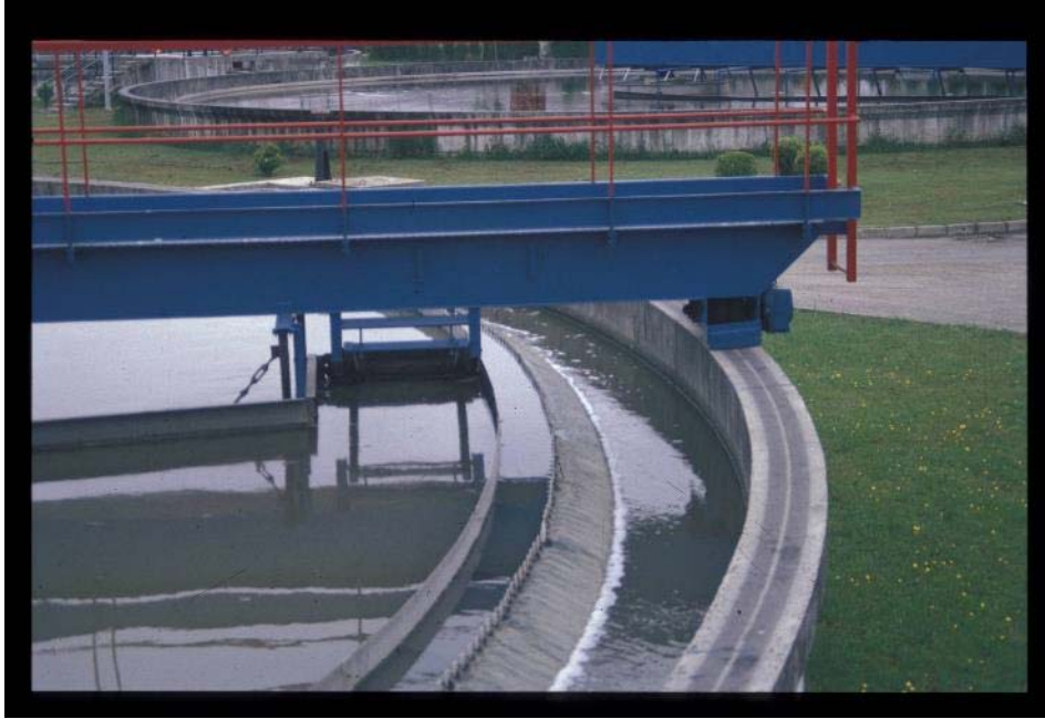
Figure 29 General view of a weir system, peripheral baffle and skimmers leading scum to the trough
