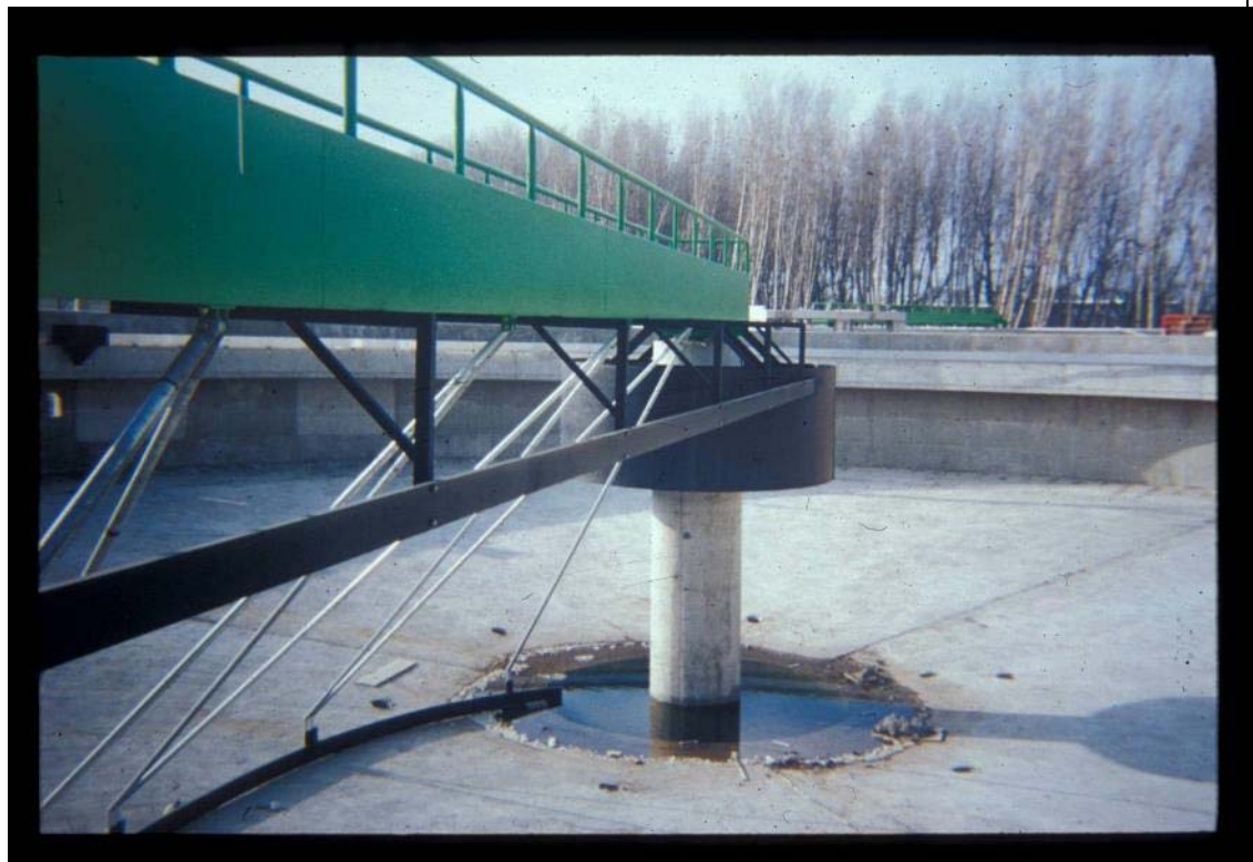
Figure 18 General view of a circular primary clarifier with moving arm and central raw water distribution system
