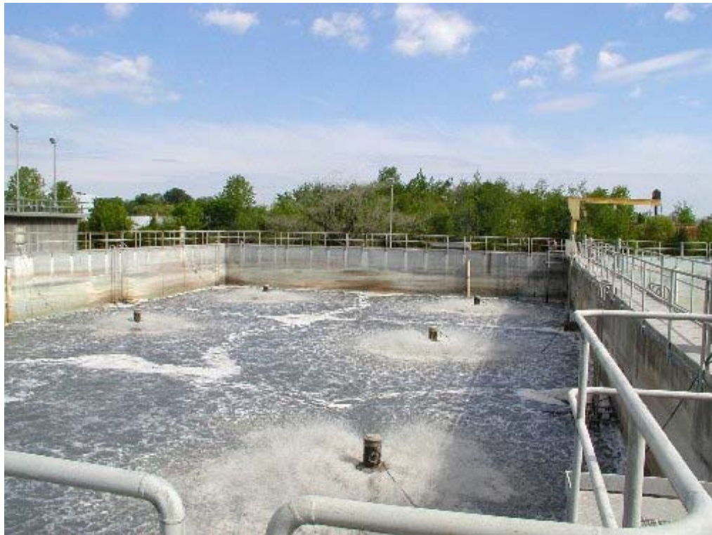
Figure 2 General image of an equalization tank with surface agitation (Cumberland County, USA).
