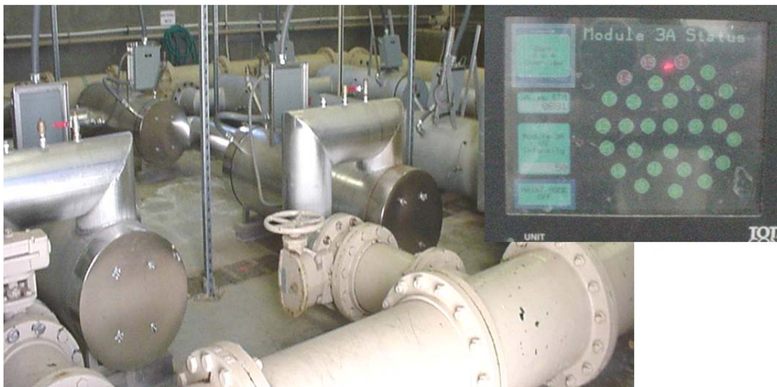
UV Trains and SCADA display.
