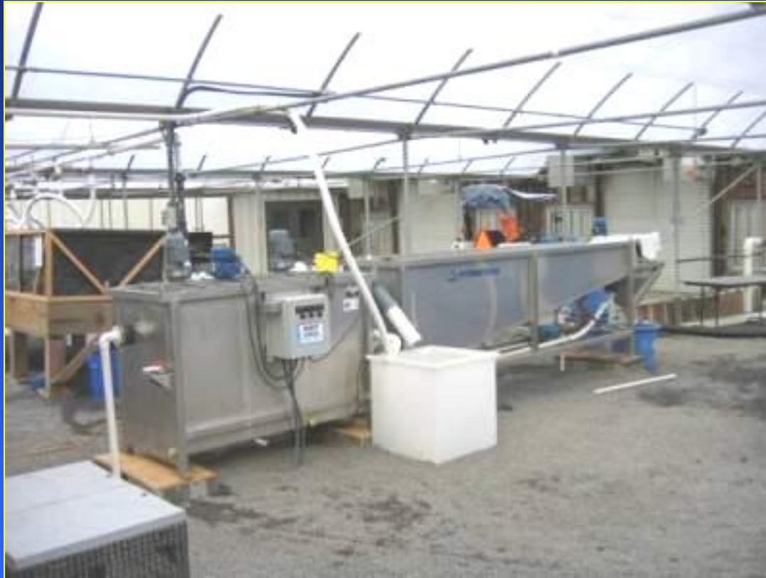
Belt Filter System, Hydrotech Model HBF537-1H
