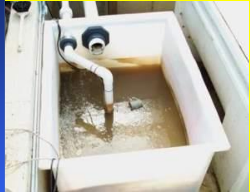
Backwash Water Sump
