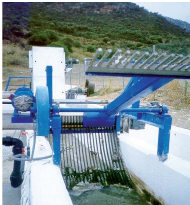
Figure 6 Curve bar screen with mechanically cleaned system
