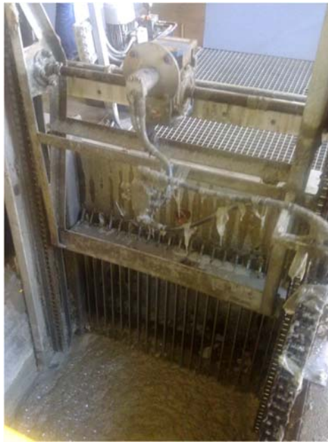
Figure 5 Coarse bar screen with mechanically cleaned system.
