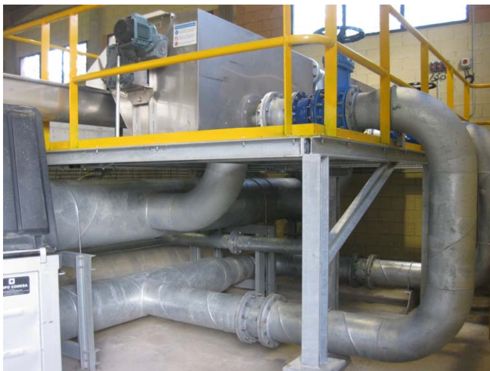
Figure 14 Detail of supply and screened water in a rotary screen.
