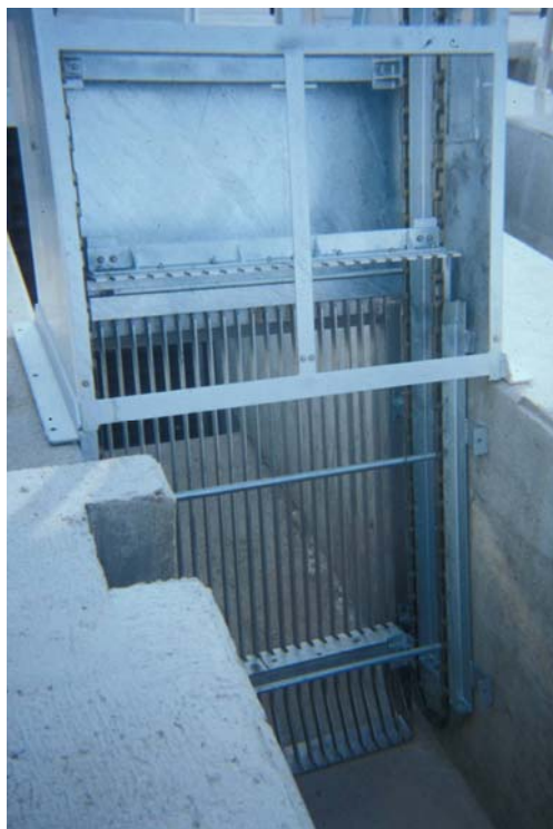
Figure 3 Coarse bar screen with coupled chain rakes cleaning system
