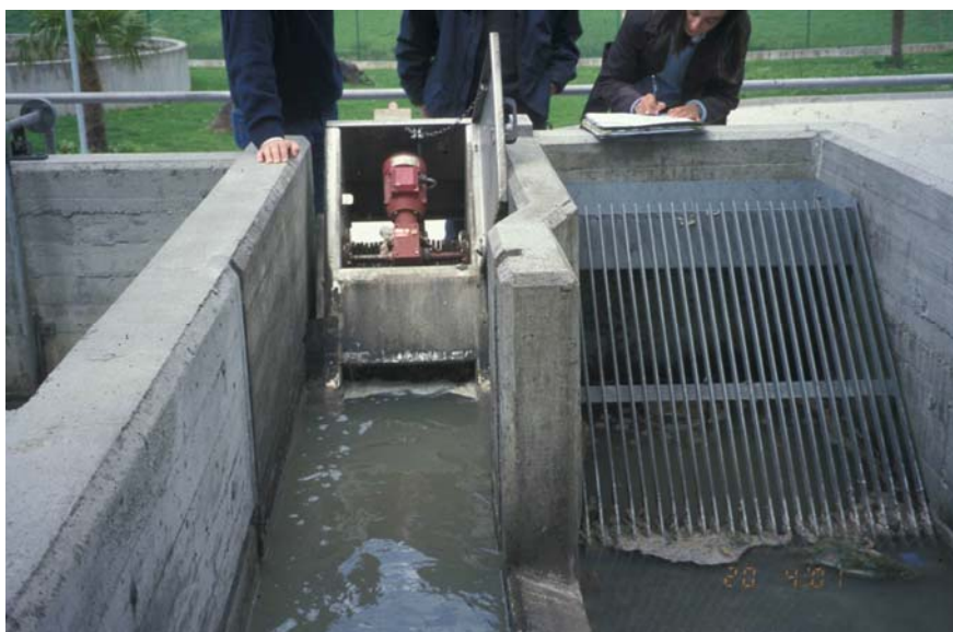
Figure 4 Double screening system. Basic hand-cleaned screen and mechanically cleaned system.
