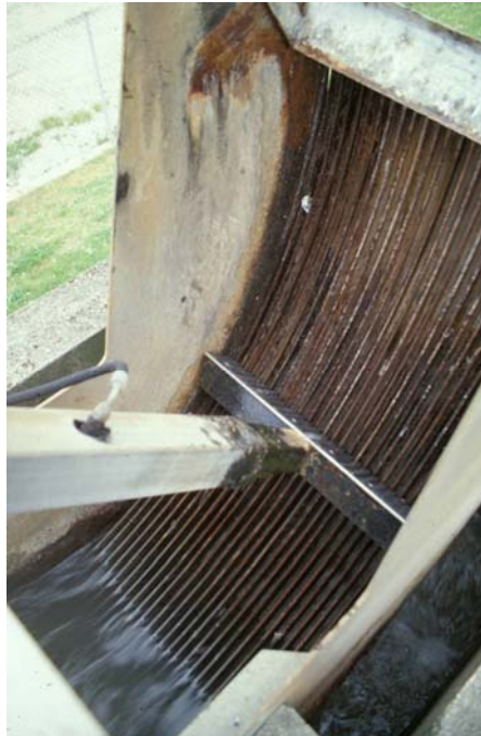
Figure 7 Fine curved bar screen with mechanically cleaned system
