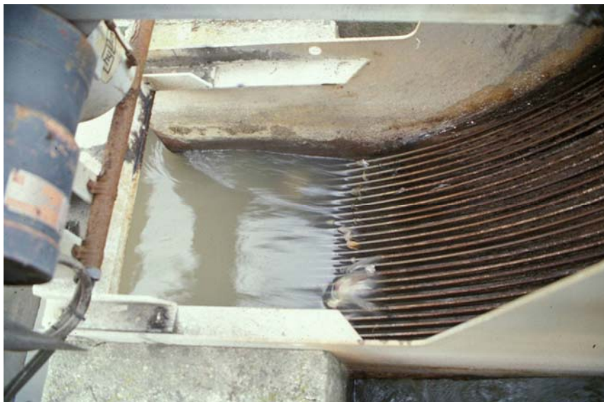
Figure 7 Fine curved bar screen with mechanically cleaned system
