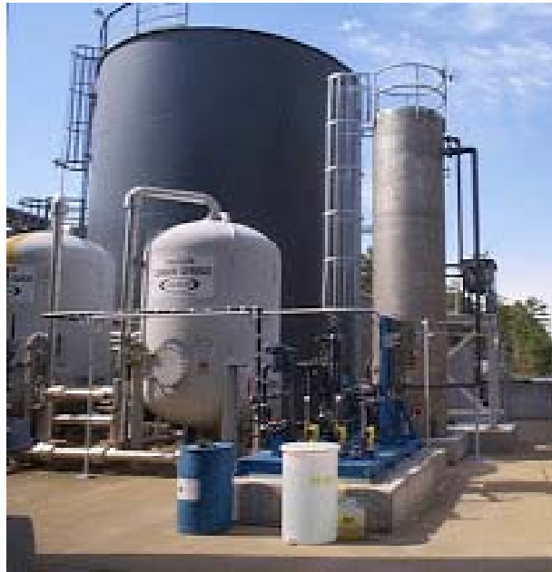
Figure 6 Fluidized bed reactors for treatment of urban or industrial wastewater, prior to activated carbon filling (Framax blog).
