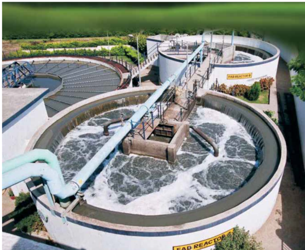
Figure 4 Aerobic fluidized bed reactors for urban wastewater treatment (Thermax system).
