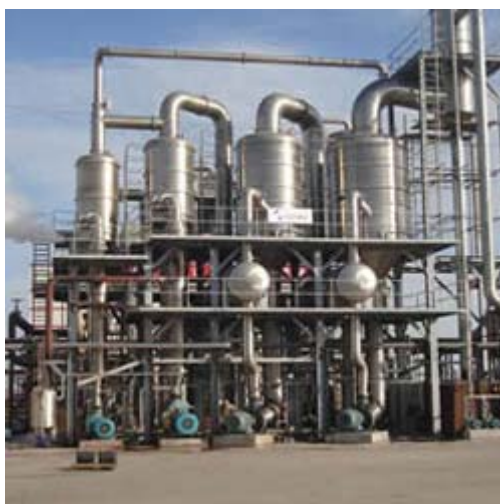
Figure 8.- Forced circulative evaporator JINZHOU GROUP CO., LTD. http://www.jzmachinery.com/IndustrialEvaporator.html (September 2015)
