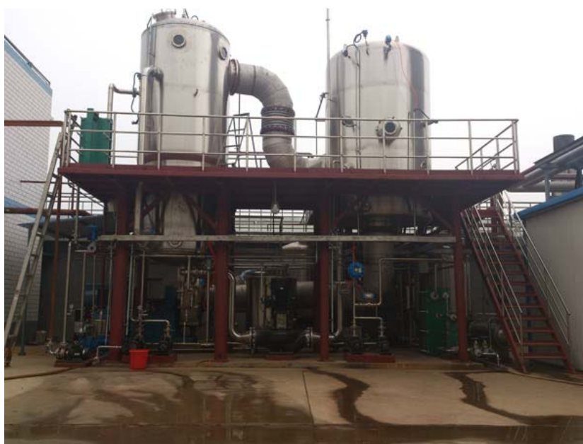
Figure 8.- General view of an evaporation installation.
