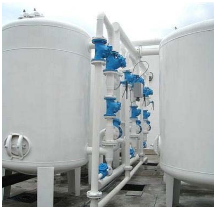
Figure 2. Industrial GAC filtration system http://www.aesasa.com.mx/
