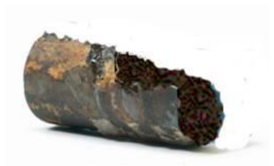
Cast Iron Pipe
