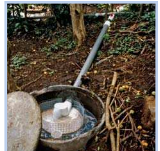
Photo 5-4: Settling tank (photo: Dallas S.)
