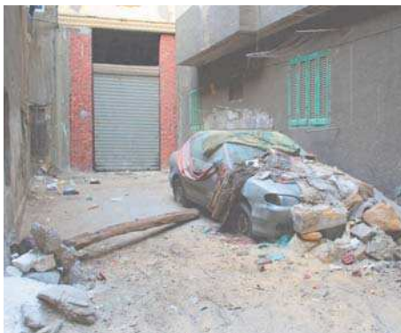
Fig. 2 Degraded buildings in El-Gamaleya
