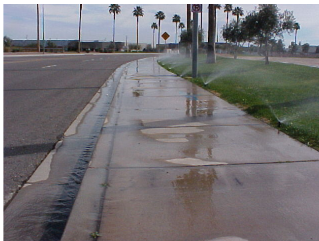
Water in the street ( Fugitive Water )
