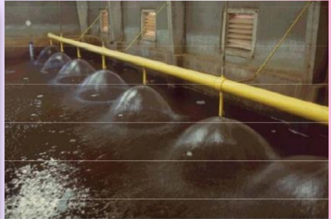
Spray Aerators: Nozzles
