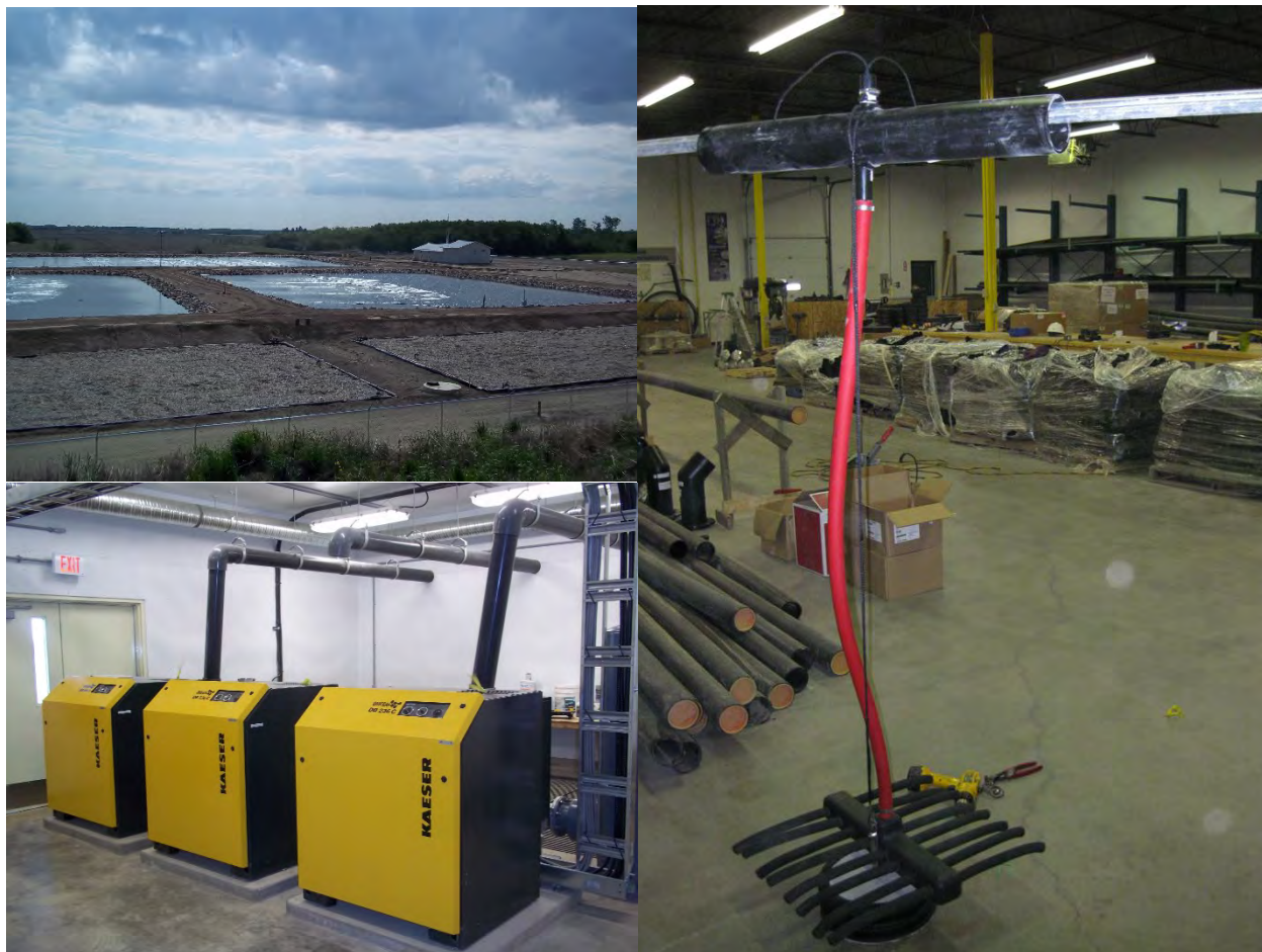
Figure 2-3 Aerated cells and SAGR (top-left), blowers (bottom left) and fine bubble diffusers (right)
