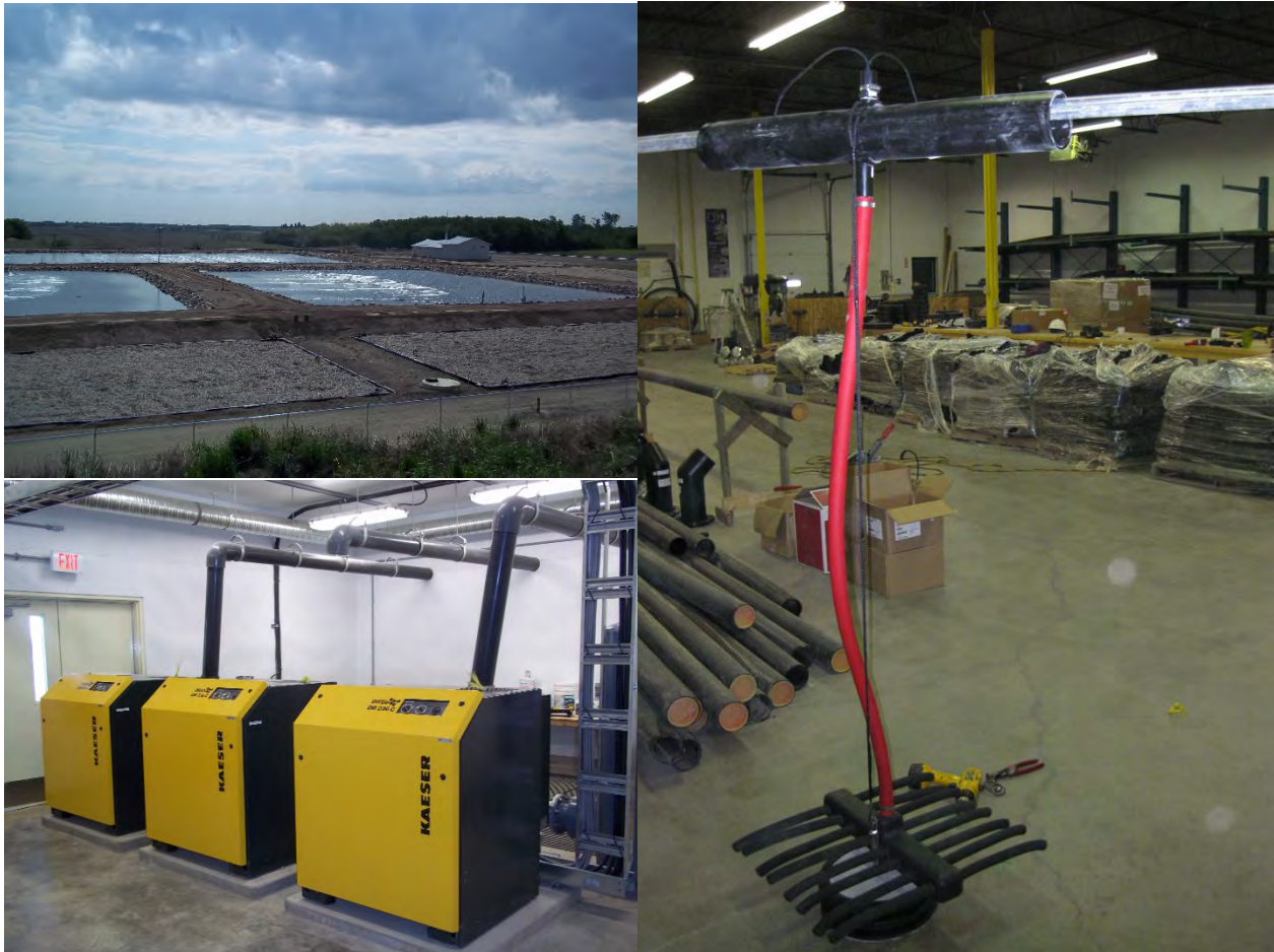
Figure 5-2 Aerated Cells and SAGR (top left), Blowers (bottom left) and Fine Bubble Diffusers (right)
