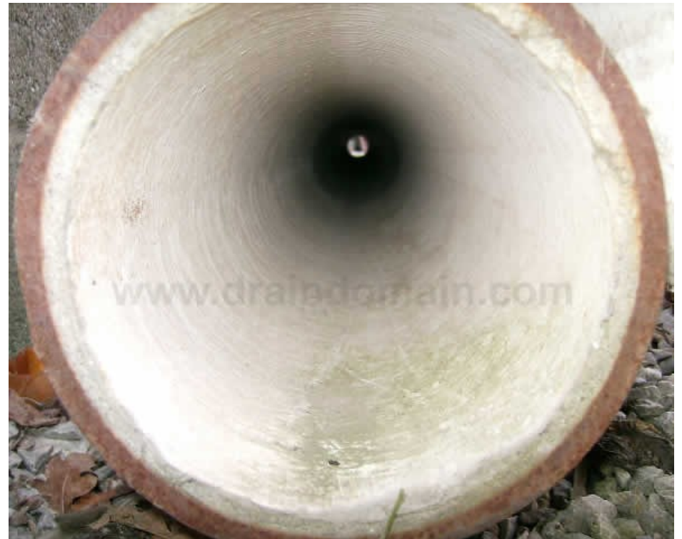
Concrete Lined Pipe
