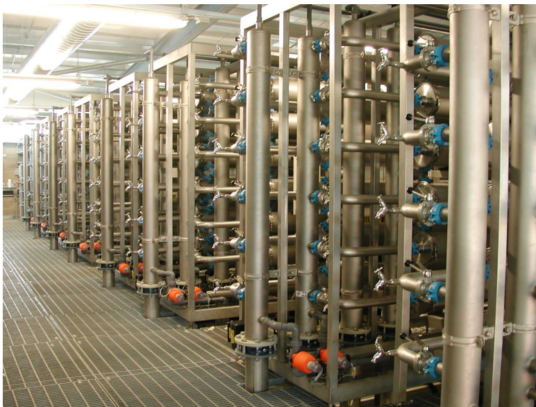
Figure 8: 6,700 \text{ m}^3\text{h}^{-1} ultrafiltration water plant.
