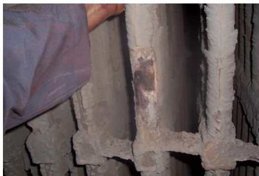
Photo 8: Fouling & corrosion over superheater
