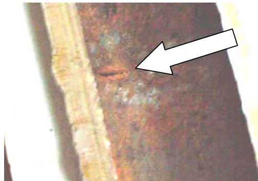
Photo 2- Failed portion from inside
