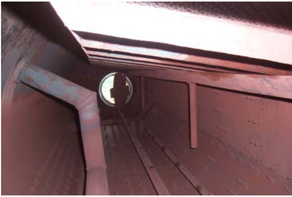
Photo 1: Chemical dosing line is laid closer to blow down line.
