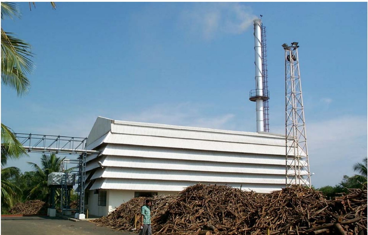
PHOTO 2: NEW WOOD FIRED BOILER
