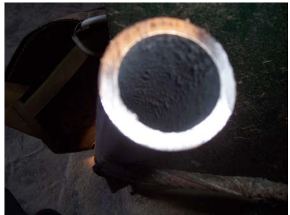
Photo 4: Deposition seen inside the SH tube, due to mechanical carryover.
