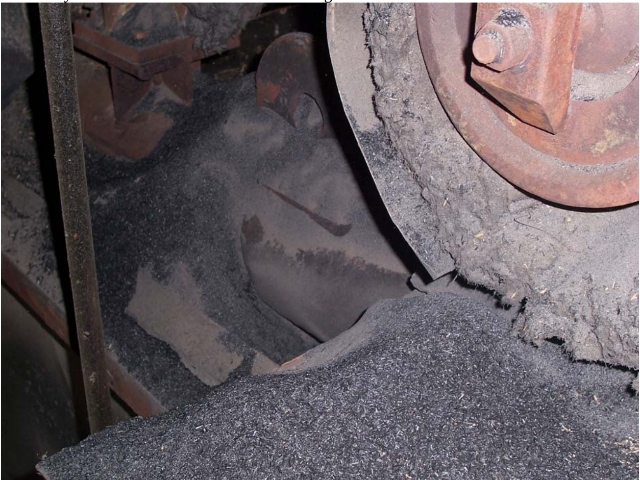
Case study 4- Photo 10: leakages around the headers.
