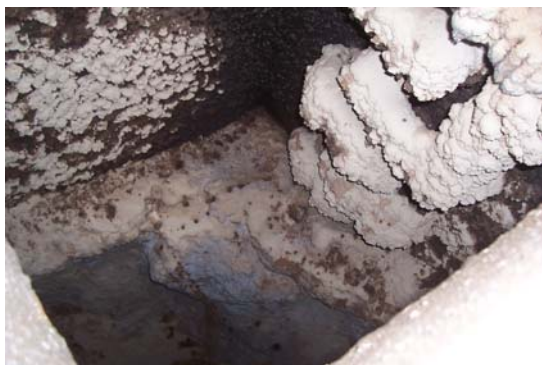
Photo 7: Ash deposition over tubes
