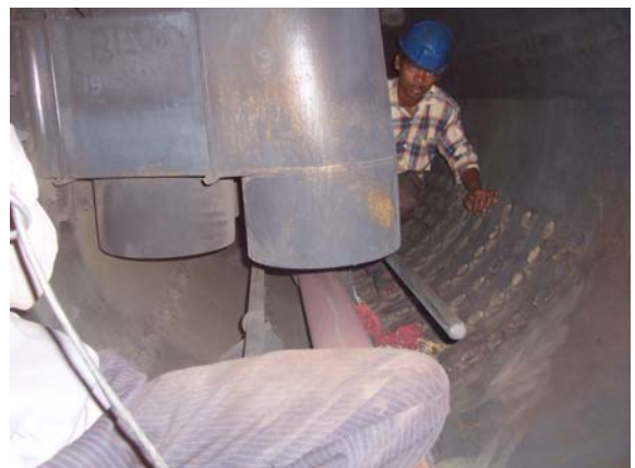
Photo 6: Drum condition with the right piping layout.
