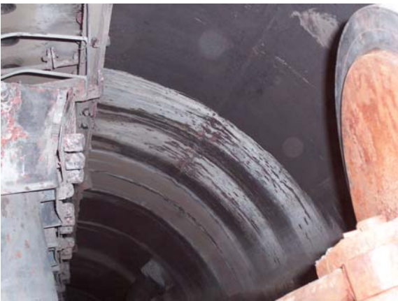
Photo 3: Physical carryover of water from cyclone separator box to drier section.
