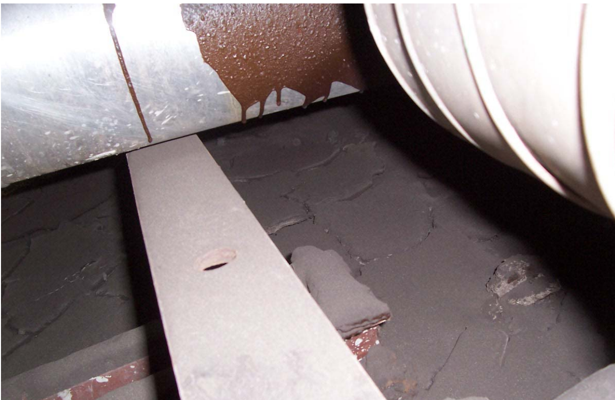
Photo 1- cracks are present in roof refractory work. Castable refractory does not arrest leaks.
