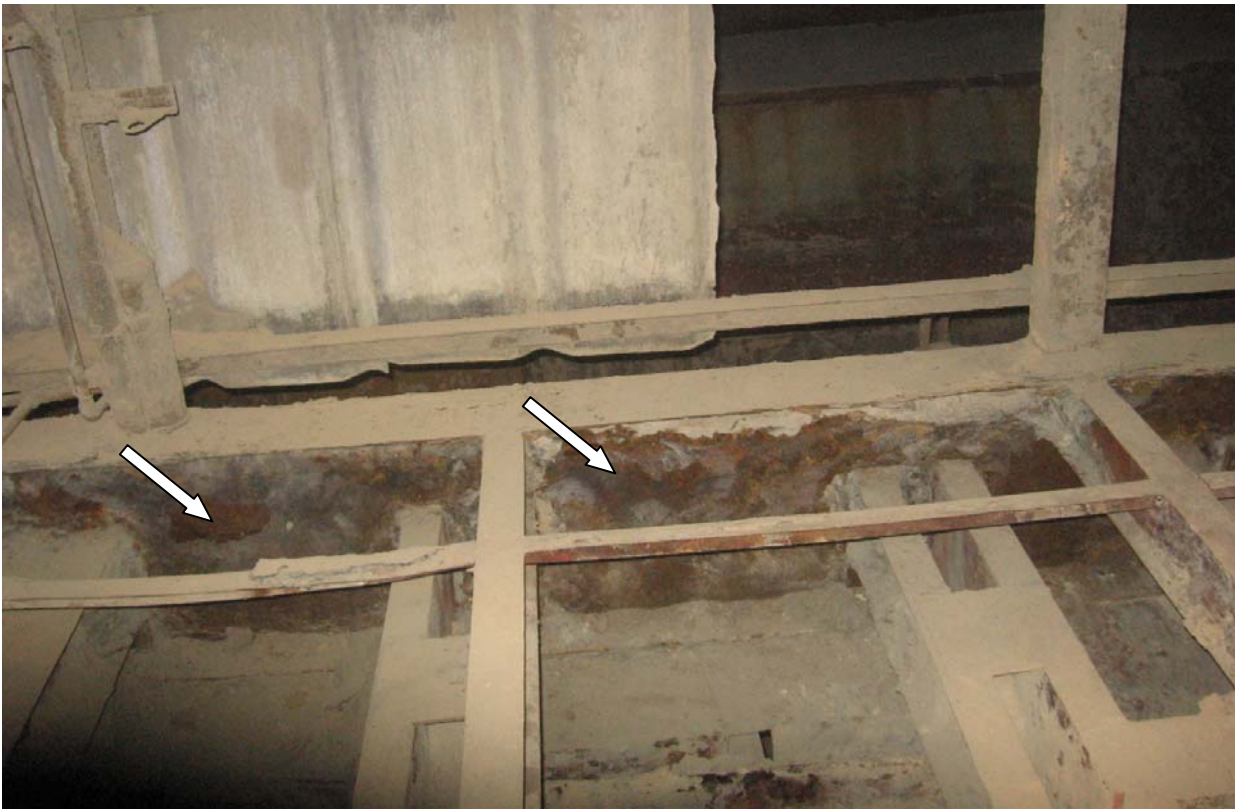
Case study 2: Photo 5- Roof beams under corrosion.
