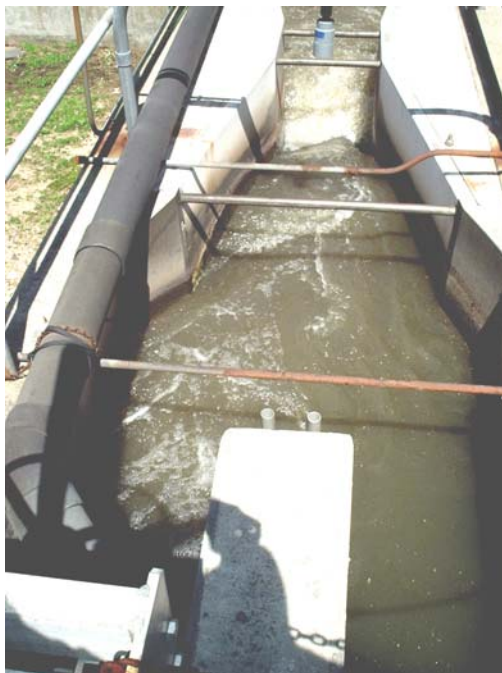
Figure 5.9 – What is wrong? 7
