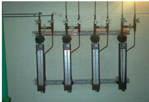
Figure 2.26 – Set of Four Venturi Flowmeters
