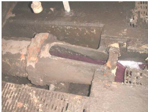
Figure 5.7 – Evidence of Surcharging by Debris on Top of the Nozzle
