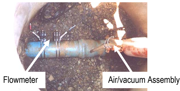
Figure 5.8 – Possible Improper Isolation Distance
