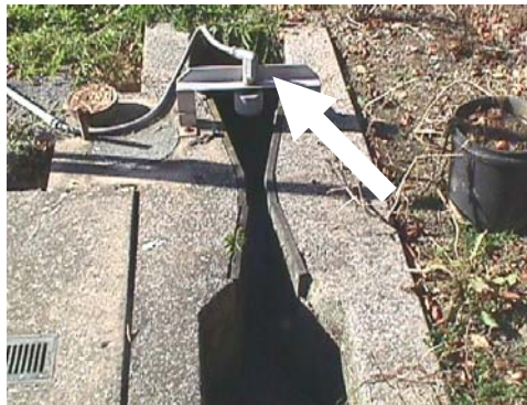
Figure 2.10 – Parshall Flume with Ultrasonic Sensor
