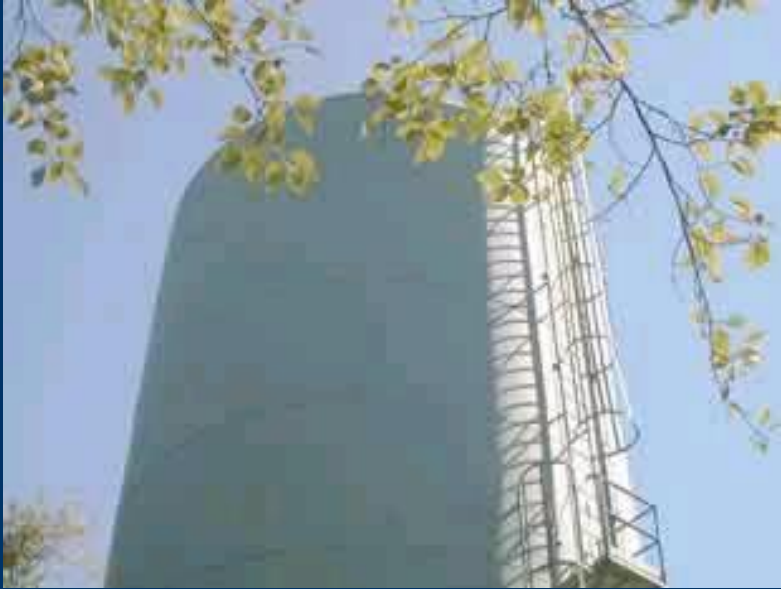
Steel water storage tank
