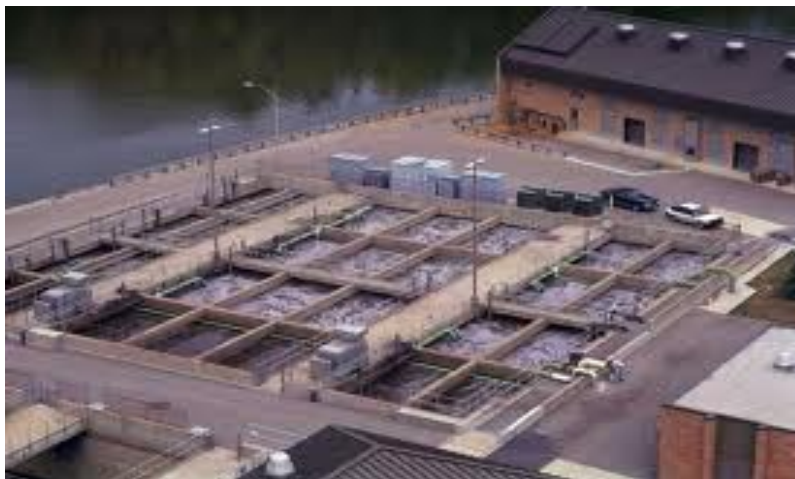
Fig 6.2: Secondary clarifier in operation.
