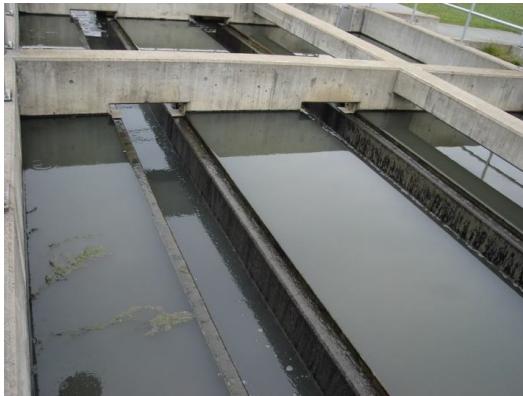
Primary Clarifier Weir
