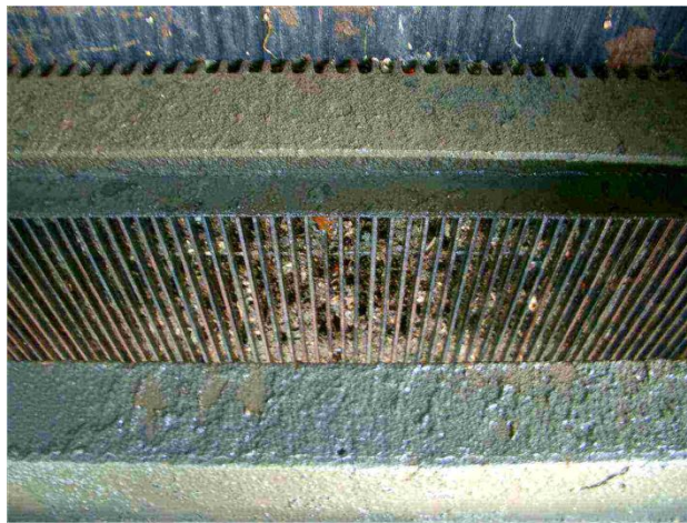
Fig 1.1 : Bar Screen in operation
