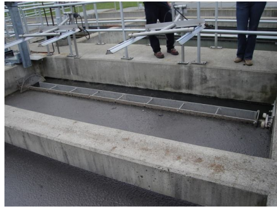
Primary clarifier scum trough
