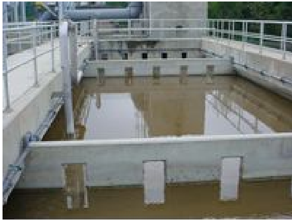
Chlorine Contact Basin
