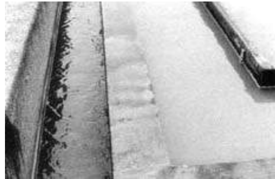
Primary Clarifier Weir
