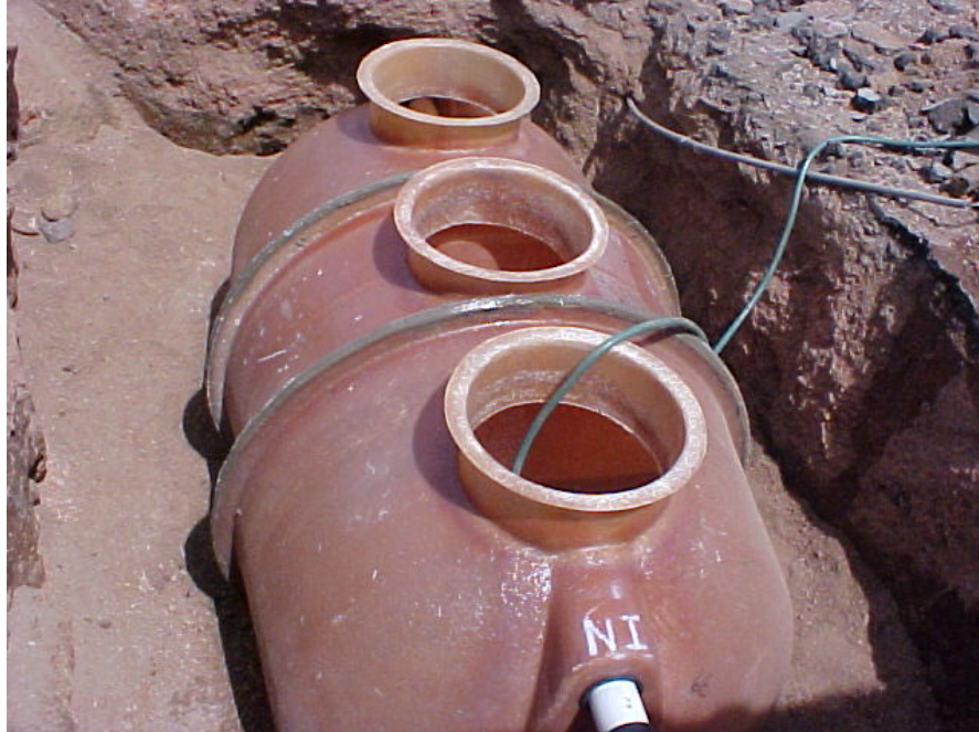
Three Compartment Grease Interceptor
