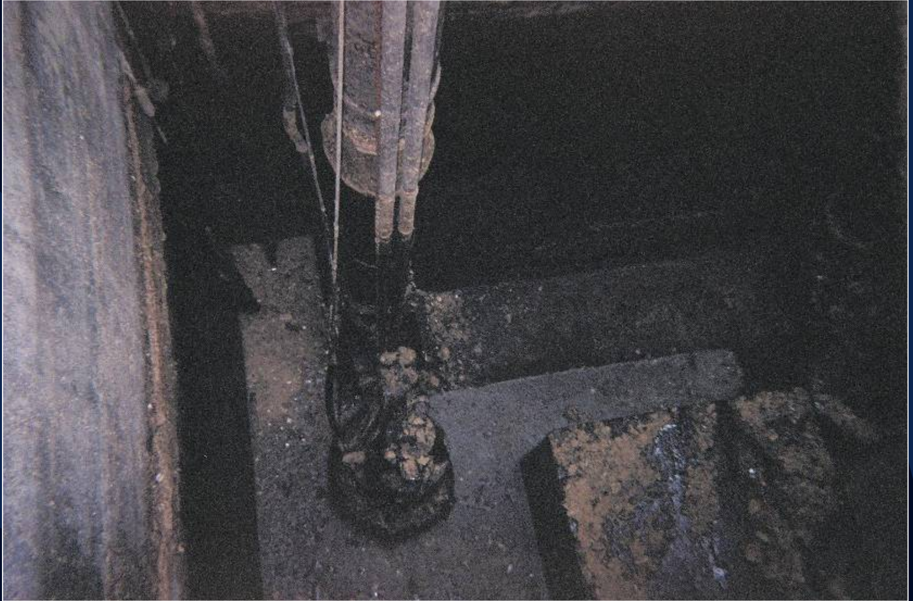
100 MGD Pump Station
