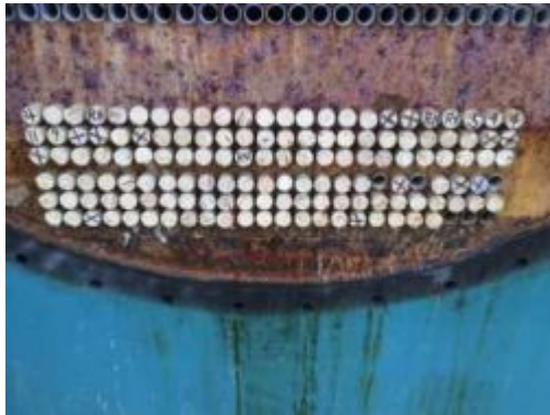
York Condenser tubes were blown from freeze damage.
