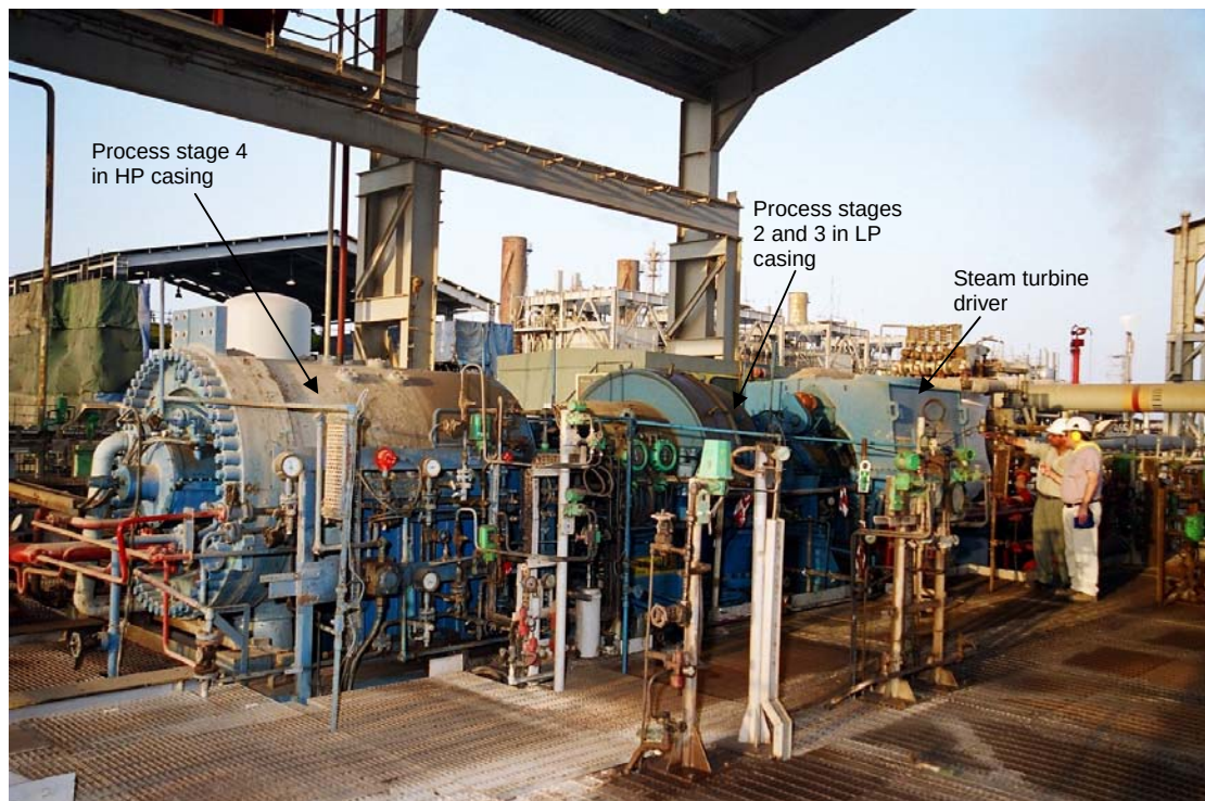
Figure 5.18: Feed-gas Compressor (Tag# 1-K-101 and 201)
