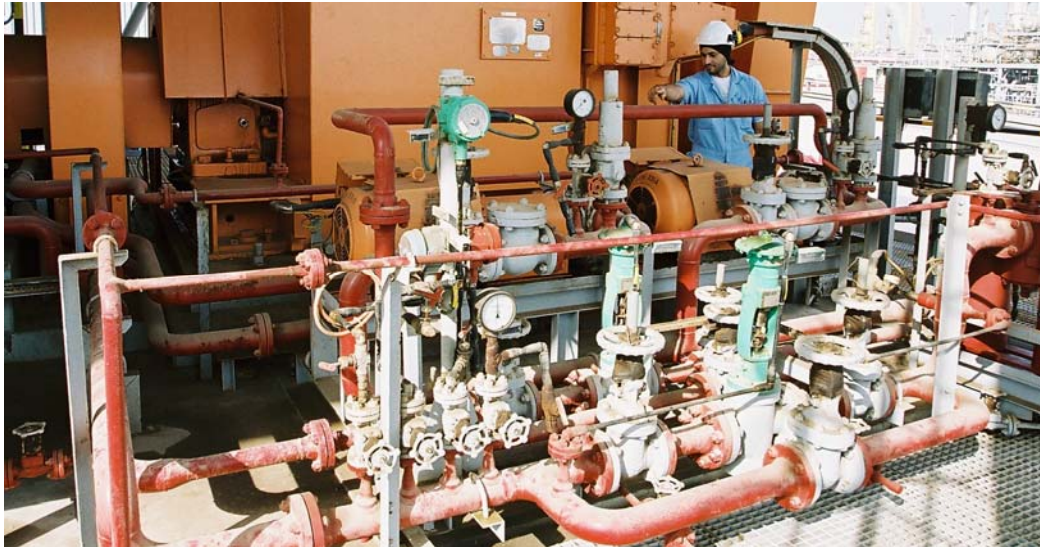
(b) Lube-oil Supply for New BOG Compressor
