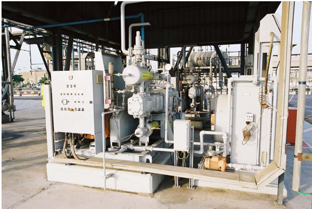
Figure 4.2: STOREX Air Compressor (Tag# 28-K-70)
