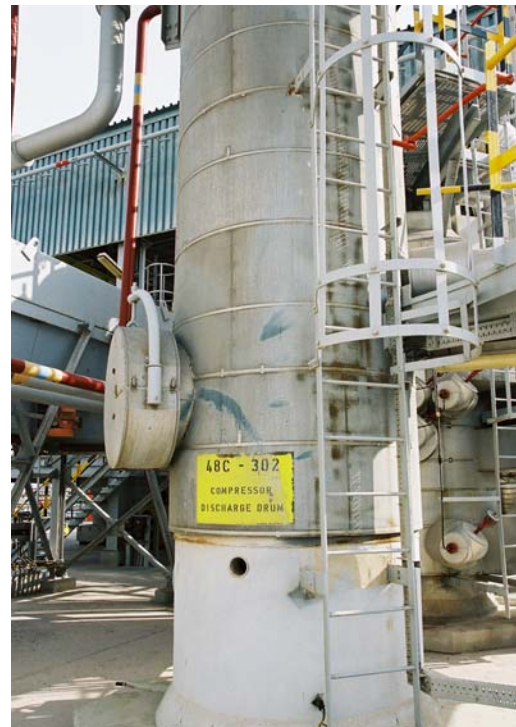
(b) Discharge Knockout Drum
