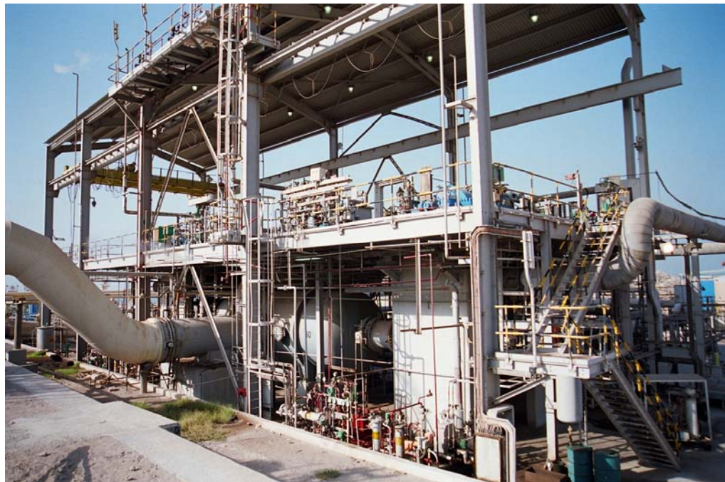
Figure 5.2: Booster Compressor Platform, Trains I and II
