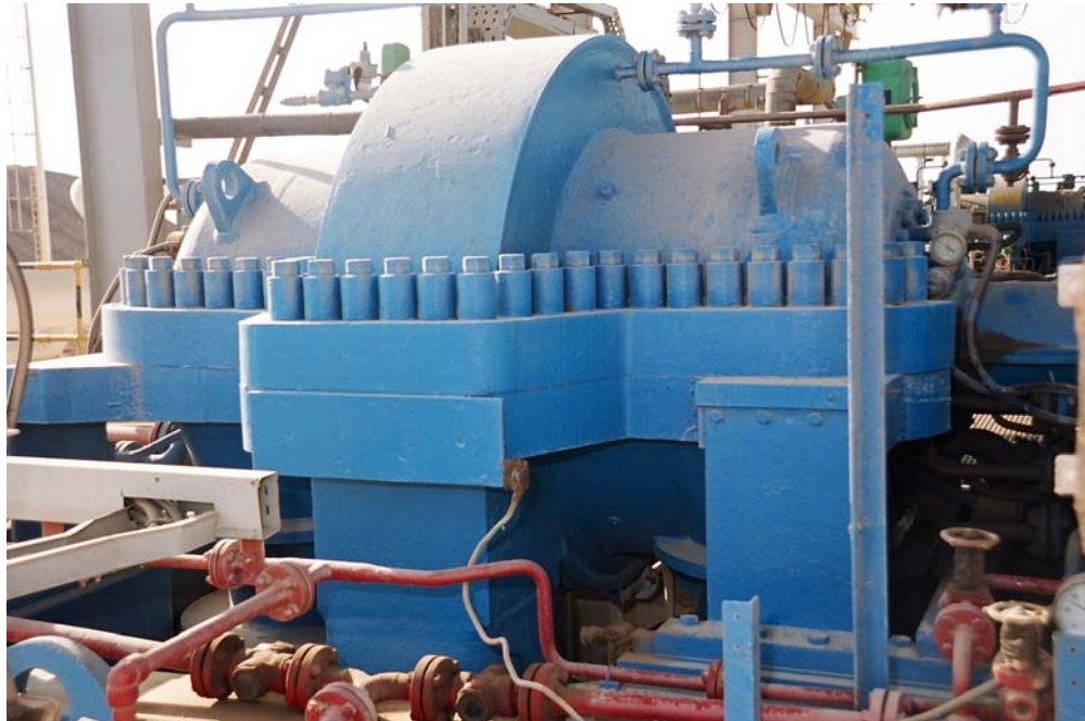
Figure 5.16: Booster Compressor (Tag# 26-K-101 and 201)
