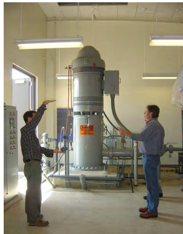
Calleguas MWD, California
