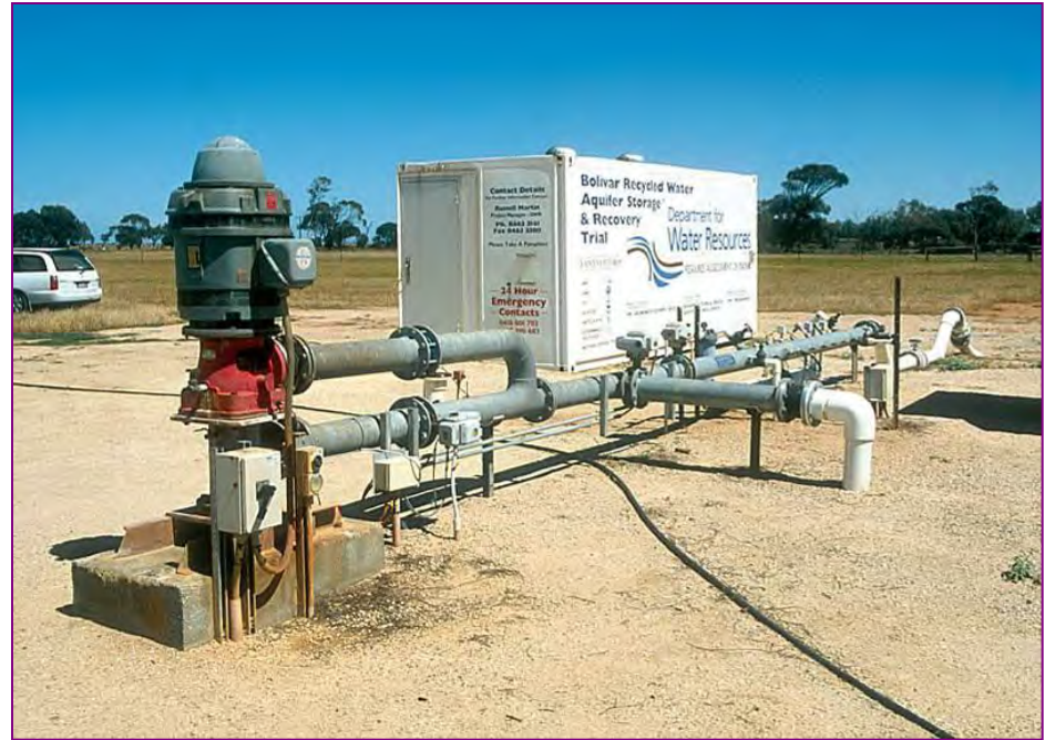
Adelaide, Australia ASR Well
