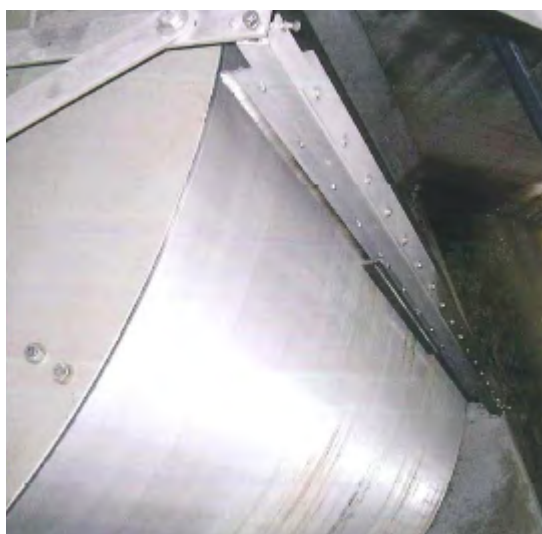
Figure 8.3 Rotary screen of the fine screen installation
