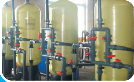
Arsenic removal plant for ground water treatment
