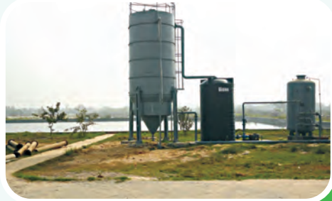
Continuous sand filter for surface water treatment
