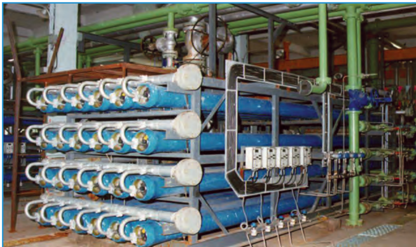
Fig 11.7 - Photograph of fully assembled RO skid
