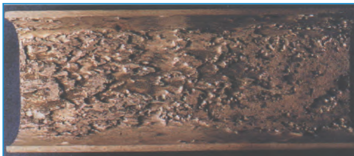
Fig 10.7 - Photograph of boiler tubes with deposits
