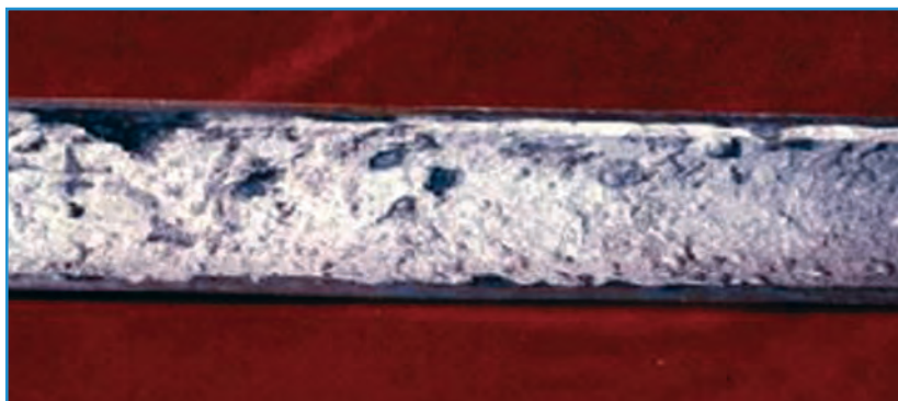
Fig 10.6 – Photograph of severely scaled boiler tube
