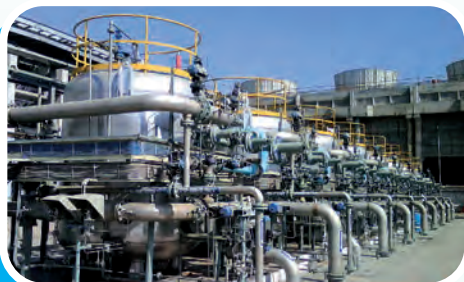
Demineralisation plant for a refinery project
