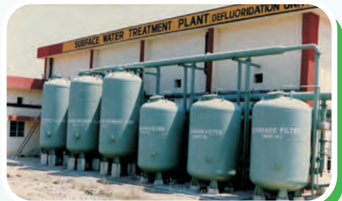
Fluoride removal plant for community drinking water systems
