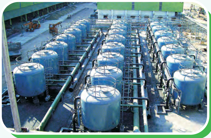
Dual media filtration for a steel plant
