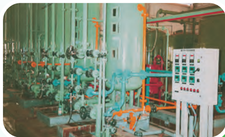
Softening plant at a sugar mill
