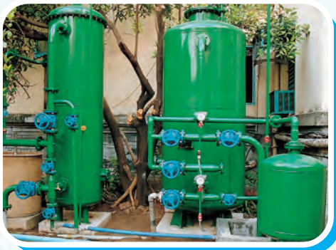
Iron removal & softening system for housing society
