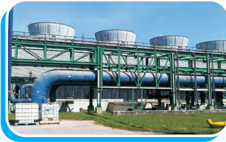
Cooling water treatment
