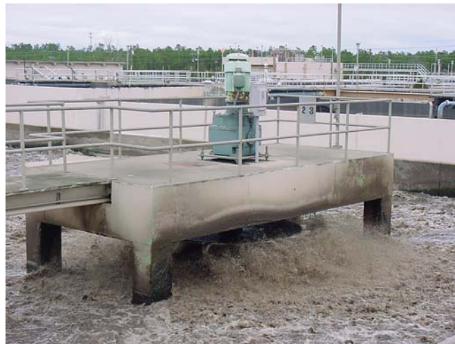
Figure 4: Mechanical aeration unit
