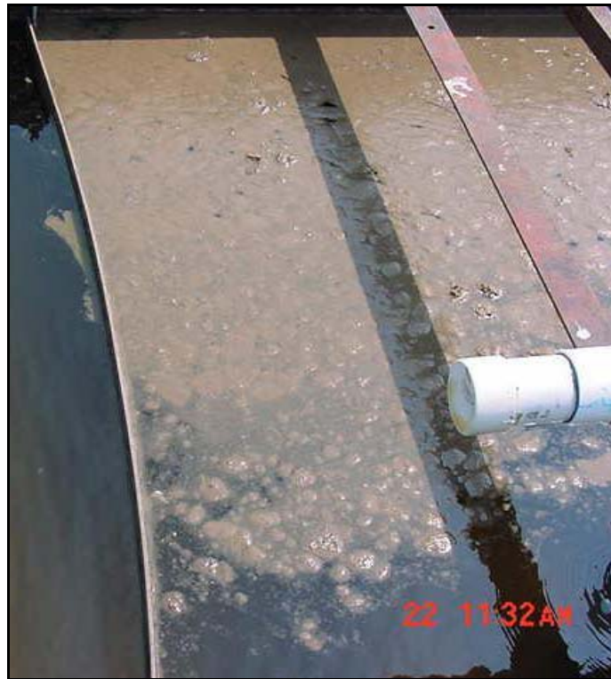
Figure 9: Light scum on clarifier surface
