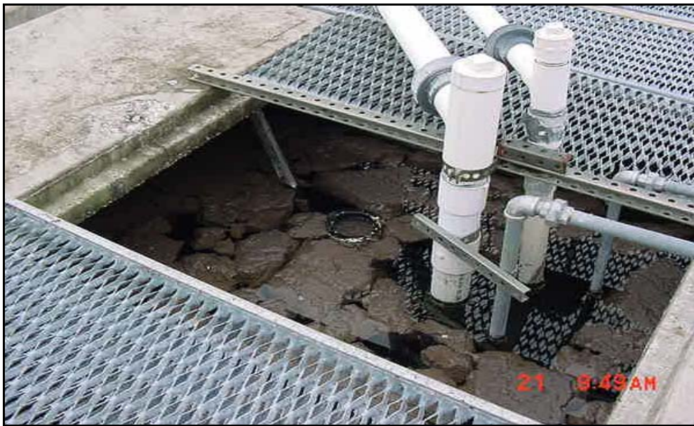
Figure 7: Rising sludge 'pop-ups' on small plant clarifier
