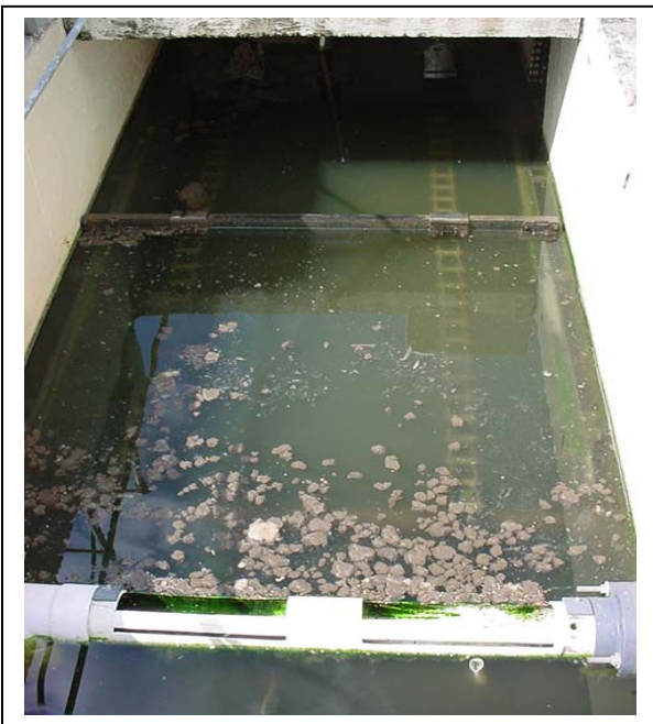
Figure 6: sludge pop-ups in a small plant clarifier
