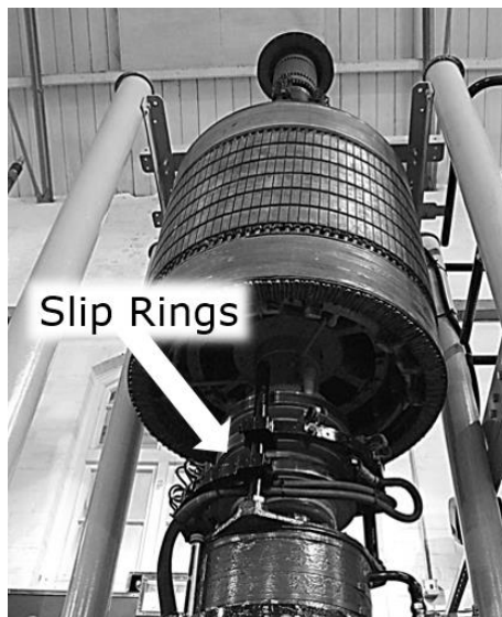
Figure 3: Rotor of induction motor with slip-rings (2)
